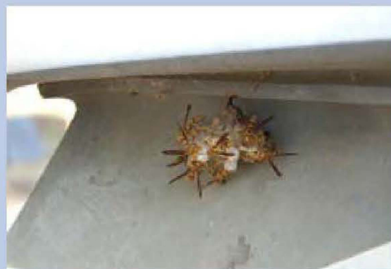
Figure D. Yellow jackets that are nesting below the projecting molding of this grave marker pose a hazard to visitors and staff because, if disturbed, they will vigorously defend their nest. Yellow jacket, paper wasp and hornet nests should be removed from grave markers by trained staff or specialists. Photo: Jason Church.
