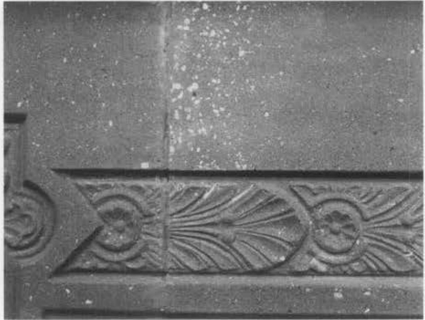
Figure 17. Unlike natural stone, cast stone generally may not be tooled in place to reduce lippage of uneven surfaces at joints. Tooling often exposes coarse aggregate from below the surface.
