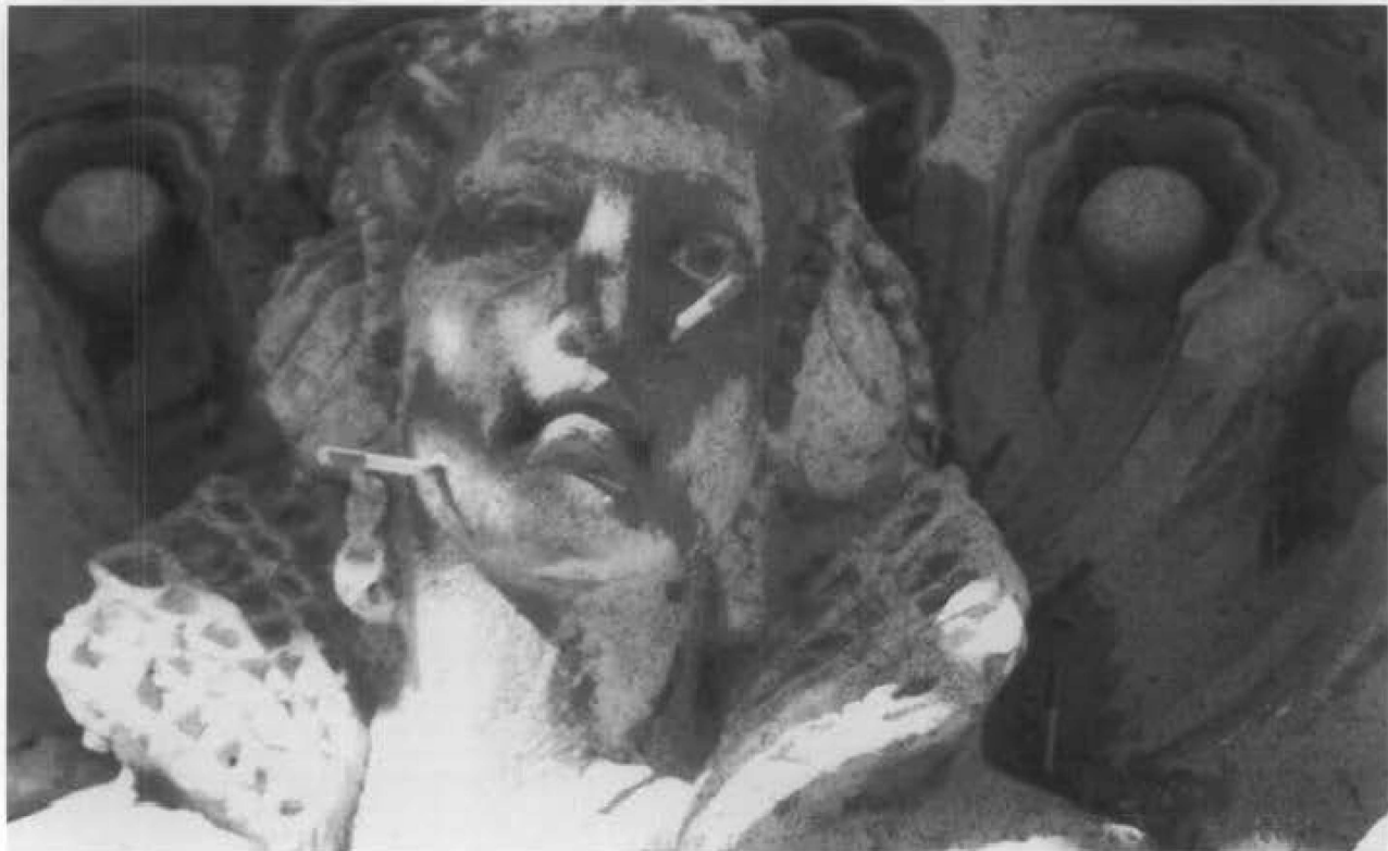
Figure 15. A delaminated layer of ornamental cast stone on the Orpheum Theater, San Francisco, California (1925), was successfully re-attached using epoxy. The multiple delivery ports for the epoxy are removed after treatment and the holes patched. Photo: David P. Wessell.
