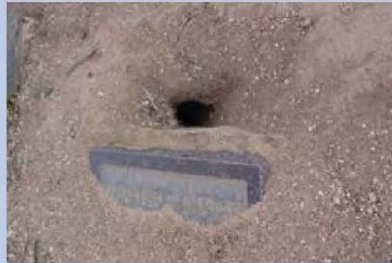
Figure C. Gophers and other burrowing animals produce uneven ground and holes that are trip and falling hazards to visitors and staff of historic cemeteries. Photo: Jason Church.
