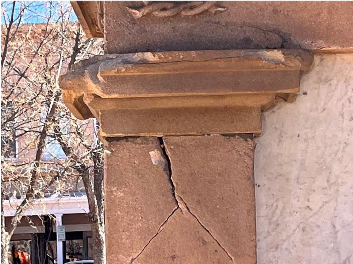
Photo 13: North elevation. Cracking of northwest pilaster. Camera facing south. March 16, 2025.
