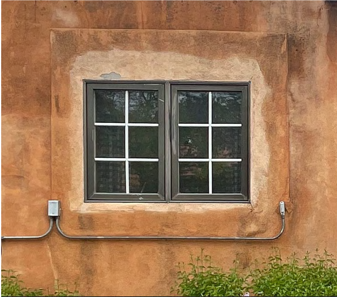
Photo 11: West elevation. Altered window at kitchen. Camera facing east.
