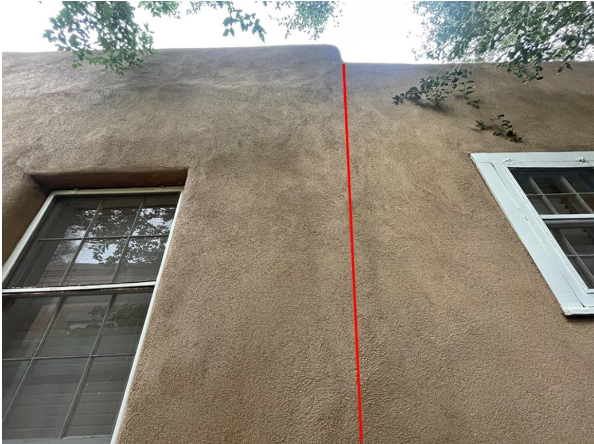
Photo 16: West elevation. South section. Demarcation line between original house and post-1958 addition. Camera facing up.
