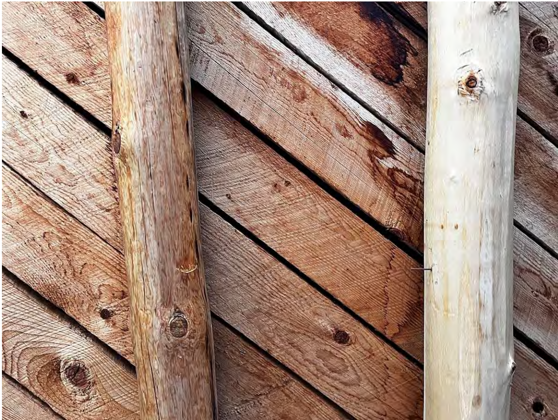
Photo 4: Porch decking. Camera facing up. October 4, 2023, JWM.
