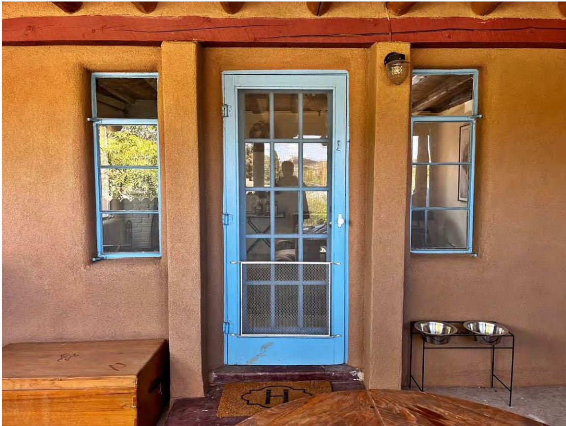
Photo 5: East elevation. Porch supports and entry door to living room. Camera facing northwest. October 4, 2023, JWM.
