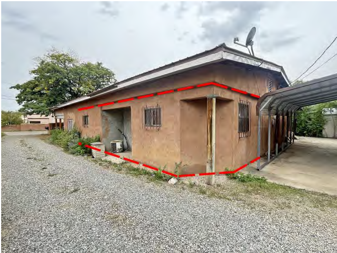
Photo 7: East and north elevations. Hatched line indicates new wall construction. Camera facing southwest.
