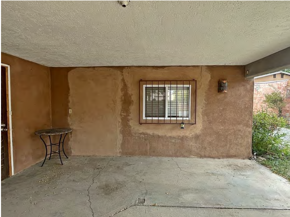
Photo 4: South (front) elevation. Porch. Note probable infilled entry door. Camera facing north.
