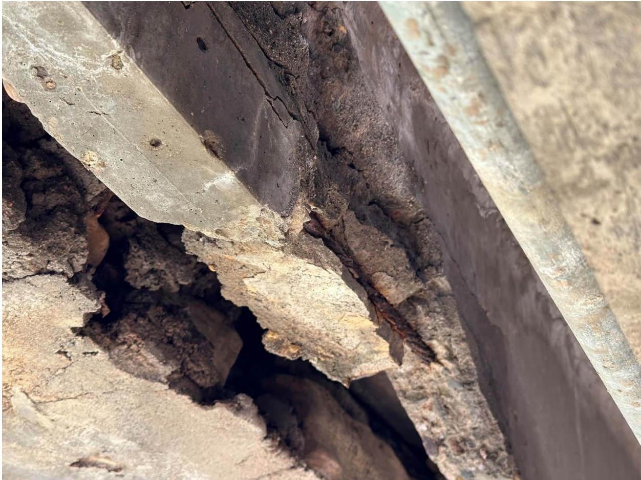
Figure 7 – Beam web spalling with exposed prestressing strand
