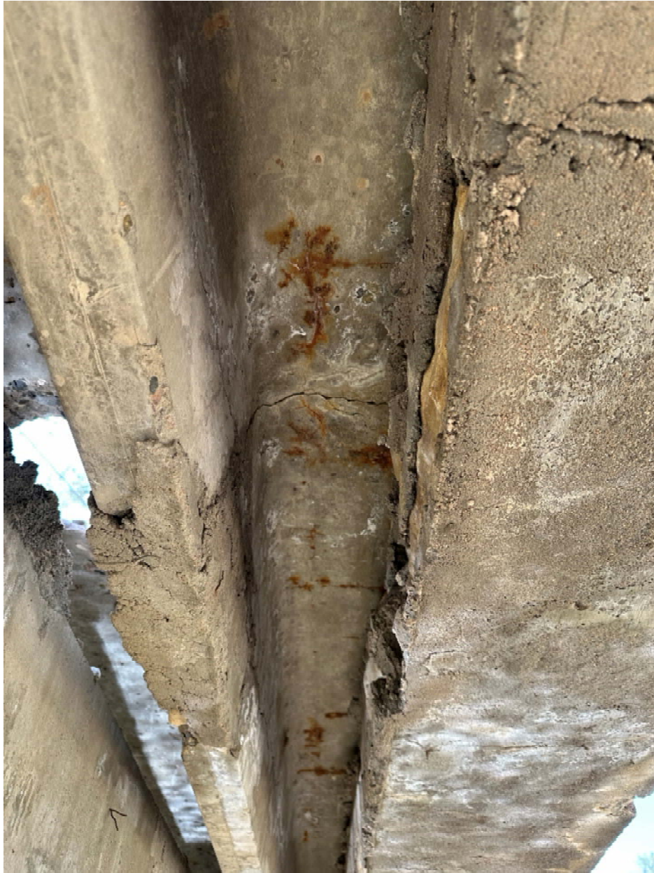
Figure 6 – Beam delamination and cracking along web and flange
