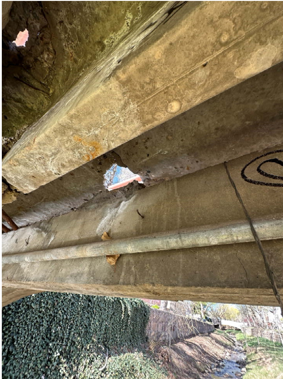
Figure 5 – Underside of flange damage
