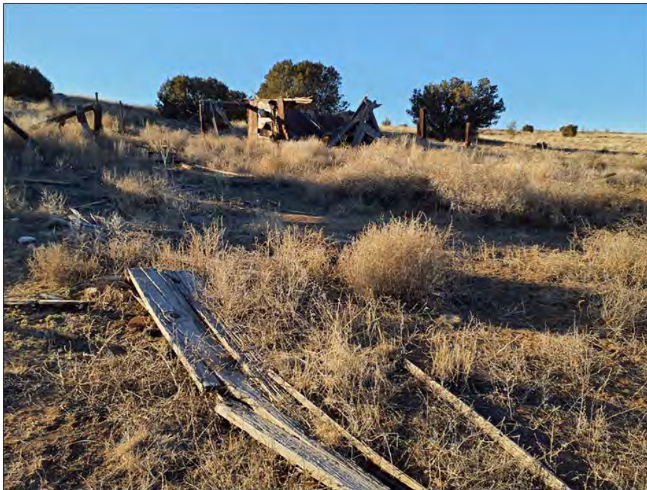
Figure 4-40. LA 54783, Feature 6 (F6), series of collapsed and partially collapsed outbuildings, corrals; view facing northwest from east side of feature (Frame T05-8232).
