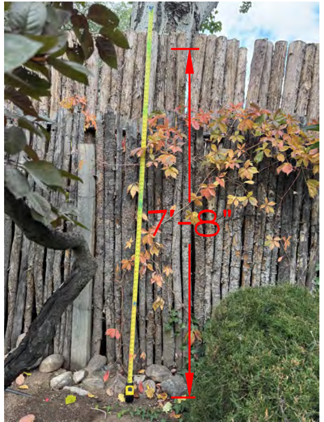
EAST FENCE FROM NEIGHBOR'S PROPERTY
