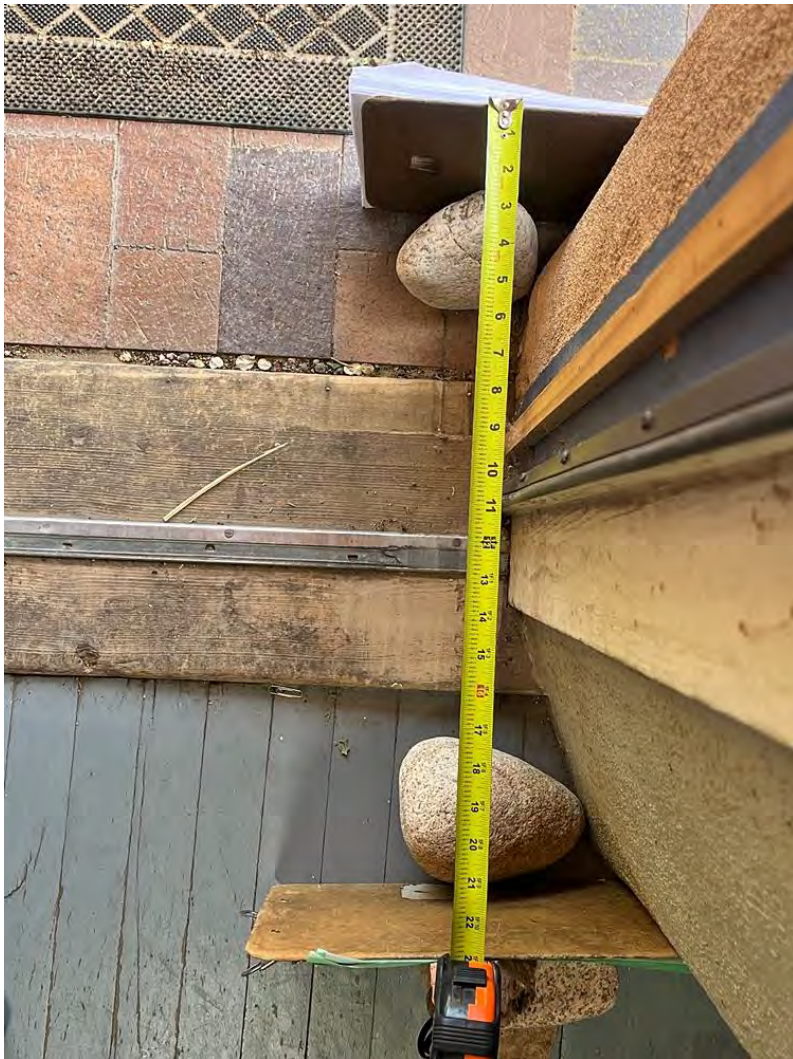
Photo 6: Primary House, north elevation. Entry door threshold. Camera facing down.
