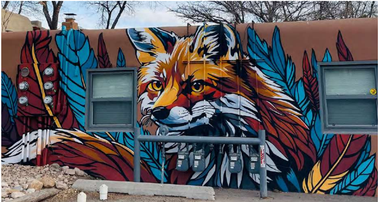
Figure 2. North publicly facing facade. The mural camouflages the existing utility boxes and lines.
