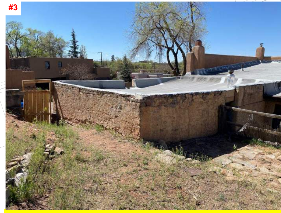
#3 RUBBLE RETAINING WALL, WATERPROOFING NOT PRESENT AND DETERIORATION PRESENTS ON EXTERIOR. THE WALL IS ALSO CONSTRUCTED WITH NON-STANDARD MASONRY MATERIAL AND PRACTICES
