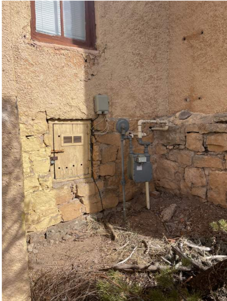
EXPOSED RUBBLE FOUNDATIONS
