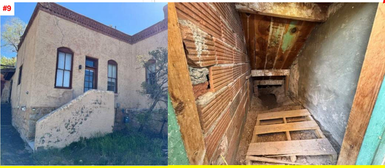
#9 PEN-TILE STAIR WALL AND WATER DAMAGE TO WOOD STAIR FRAMING, FUNGAL DECAY OF WOOD HAS BEGUN AND HAS COMPROMISED THE STRUCTURAL SECTION
