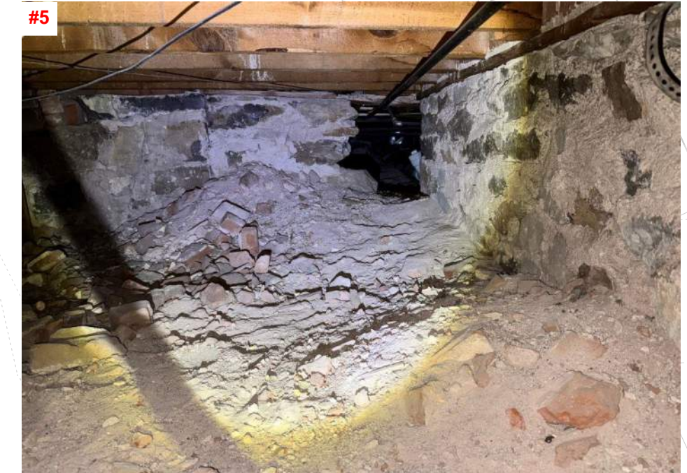
#5 PLUMBING AND HVAC ACCESS HOLES HAVE BEEN TUNNELED THROUGH THE STONE RUBBLE STEM WALL
