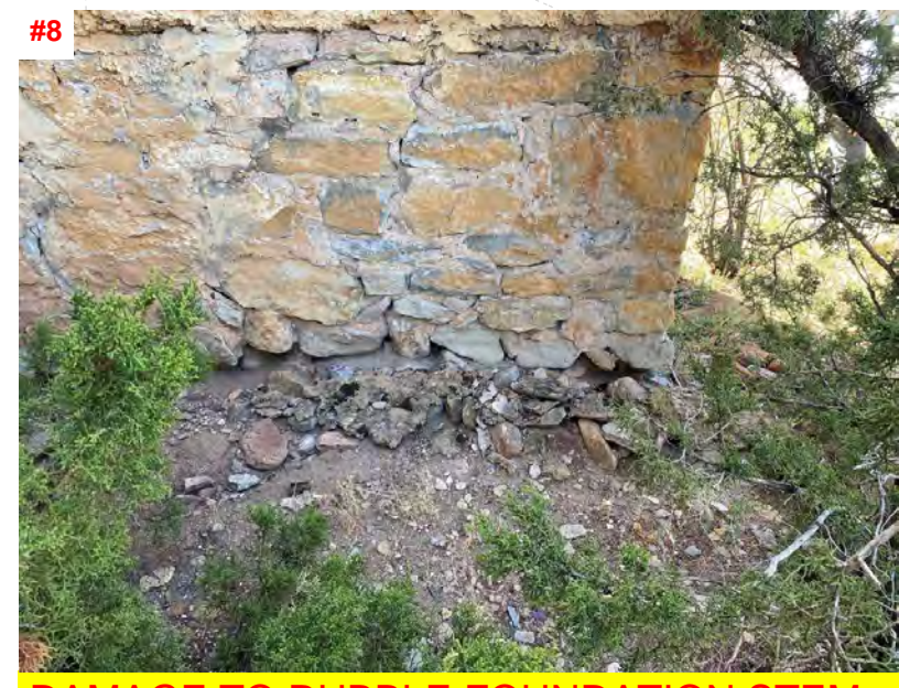
#8 DAMAGE TO RUBBLE FOUNDATION STEM WALL
