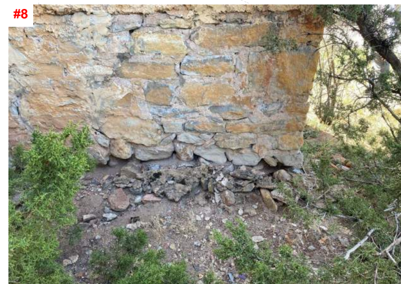
#8 DAMAGE TO RUBBLE FOUNDATION STEM WALL
