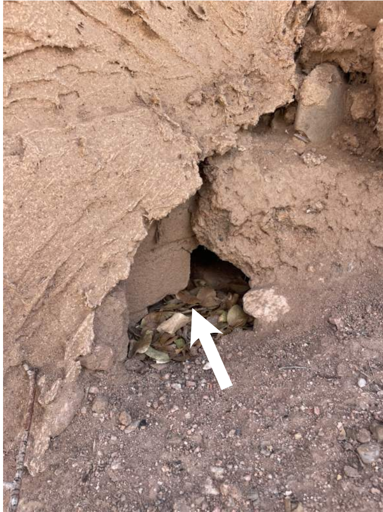
ADOBE BRICK DETERIORATING, NO FOUNDATIONS
