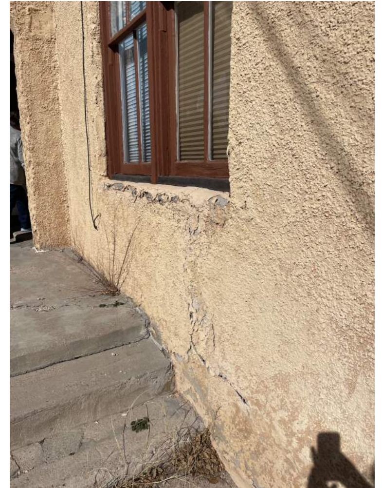
CAUSE OF CRACKS
