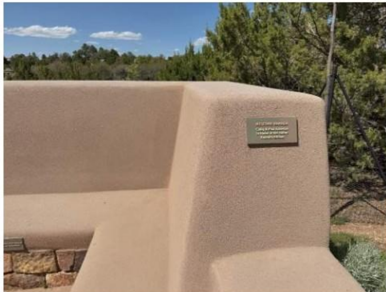
Existing integrally colored stucco site walls found in the Santa Fe Botanical Garden.
