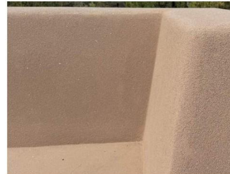
Proposed integrally colored stucco will match the color and texture of the existing Botanical Garden.
