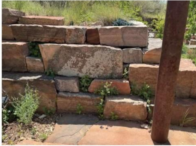
Existing moss rock masonry walls found throughout the Santa Fe Botanical Garden.
