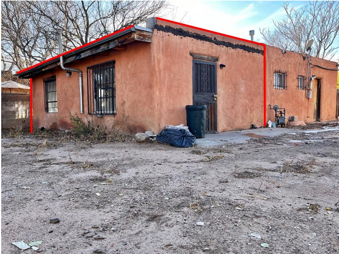
Photo 5: East and north elevations. 1980s addition outlined in red. Camera facing southwest.
