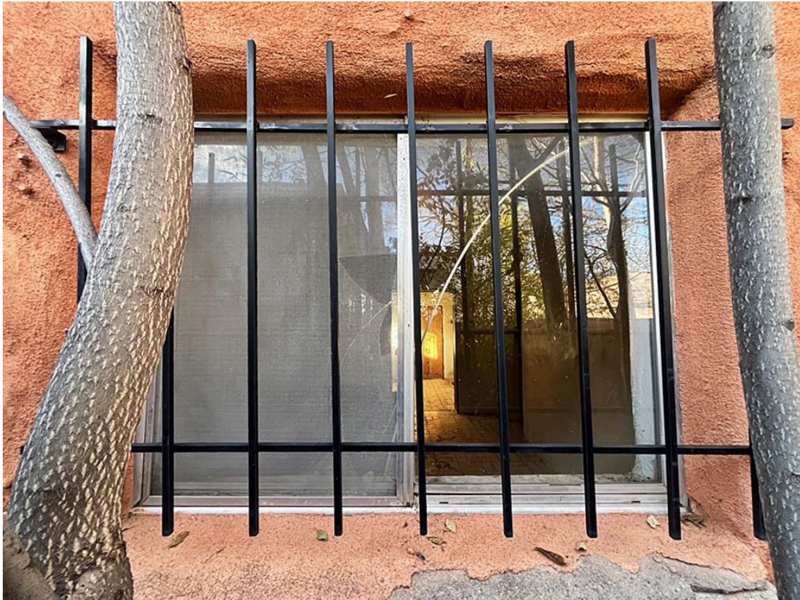
Photo 15: South elevation. Window of southwest room of the original core. Camera facing north.
