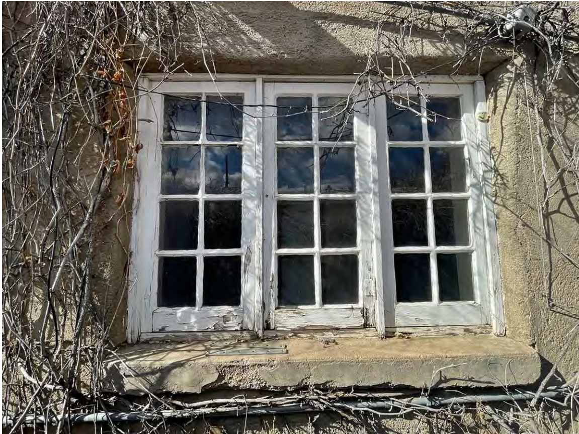
Photo 12: East elevation. Windows at southeast corner. Camera facing west. Michael Zimmer, January 29, 2025.
