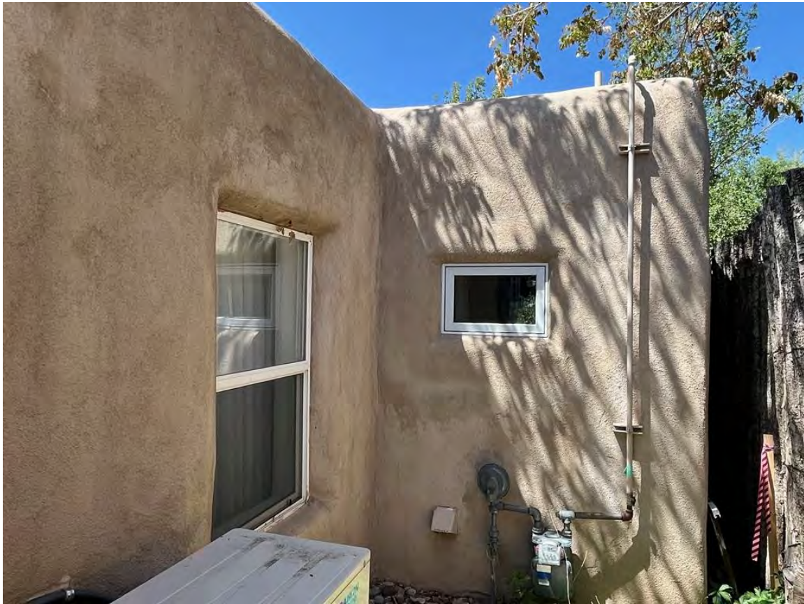
Photo 11: East elevation, south end. Windows in original garage and 1940s addition. Camera facing northwest.
