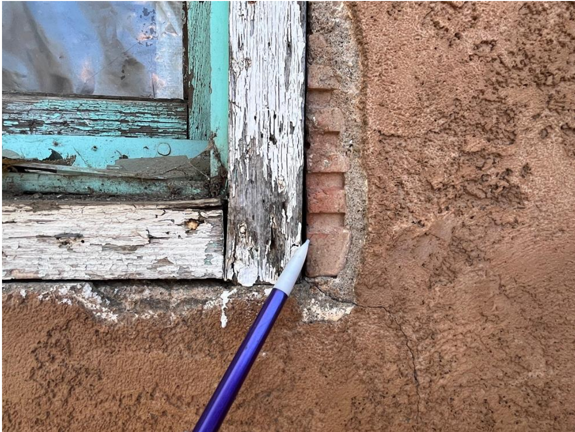
Photo 37: Building #3. North elevation. Window east of chimney. Clay tile block construction exposed. Camera facing south.
