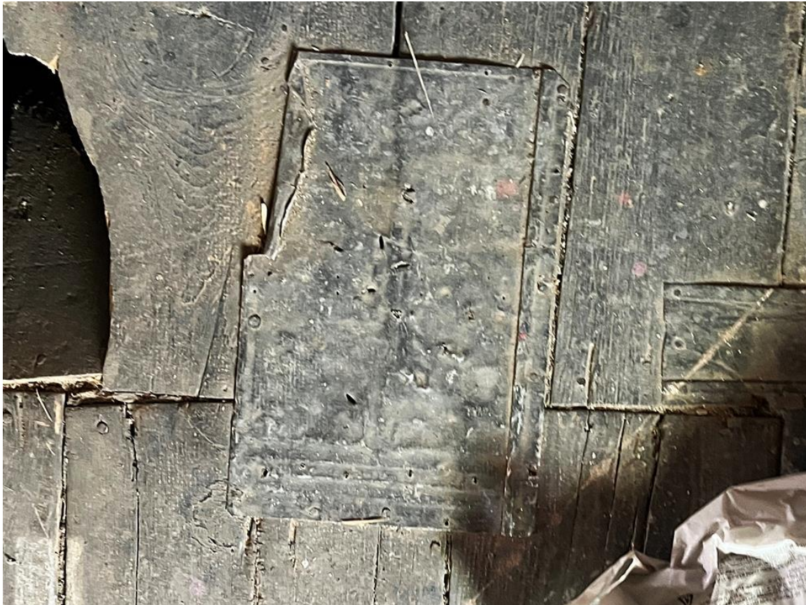
Photo 18: Building #1. Interior of southwest room. Homemade mending plate. Camera facing down.
