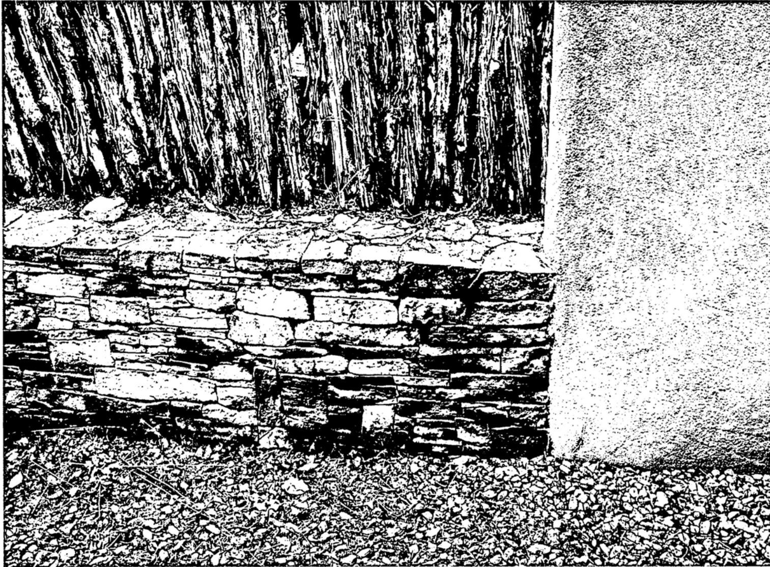
VIEW OF EXISTING STONE FOUNDATION WALL WITH EXISTING COYOTE FENCE WHICH WILL BE REPLACED WITH A BLOCK WALL
