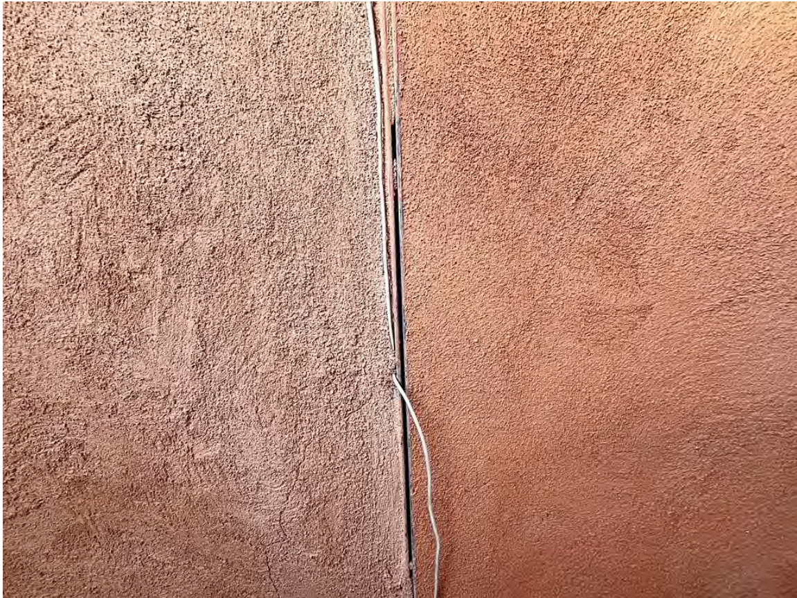
Photo 13: South elevation. Expansion joint between original core (left) and 1980s addition (right). Camera facing north.
