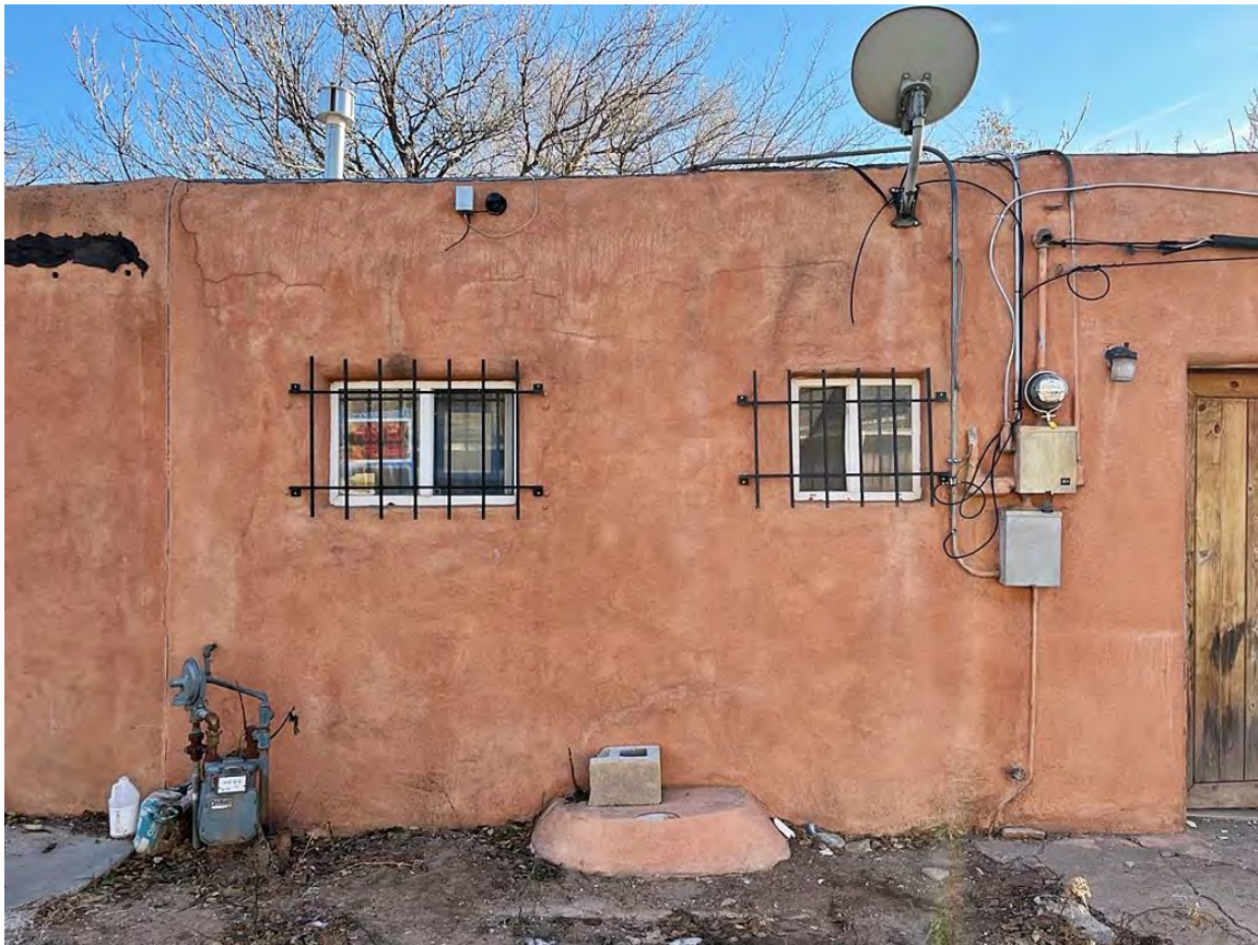
Photo 7: North elevation fenestration representing the kitchen (left) and bathroom (right) of the northeast room of the original core. Camera facing south.
