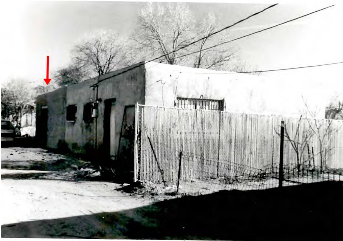
Figure 5: August 1985 HBI survey. The arrow indicates 1980s east addition. Susan Lopez, photographer. Courtesy of NMCRIS.
