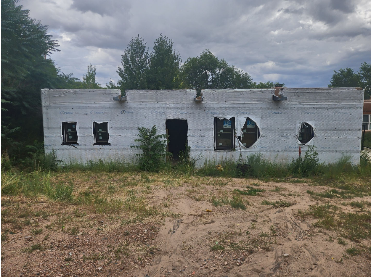
Front elevation looking west at the subject studio. Simple double hung windows replace the decrepit garage doors and a single entrance door to the artist studio.
