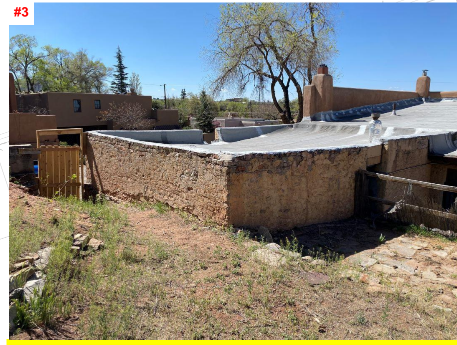
RUBBLE RETAINING WALL, WATERPROOFING NOT PRESENT AND DETERIORATION PRESENTS ON EXTERIOR. THE WALL IS ALSO CONSTRUCTED WITH NON-STANDARD MASONRY MATERIAL AND PRACTICES
