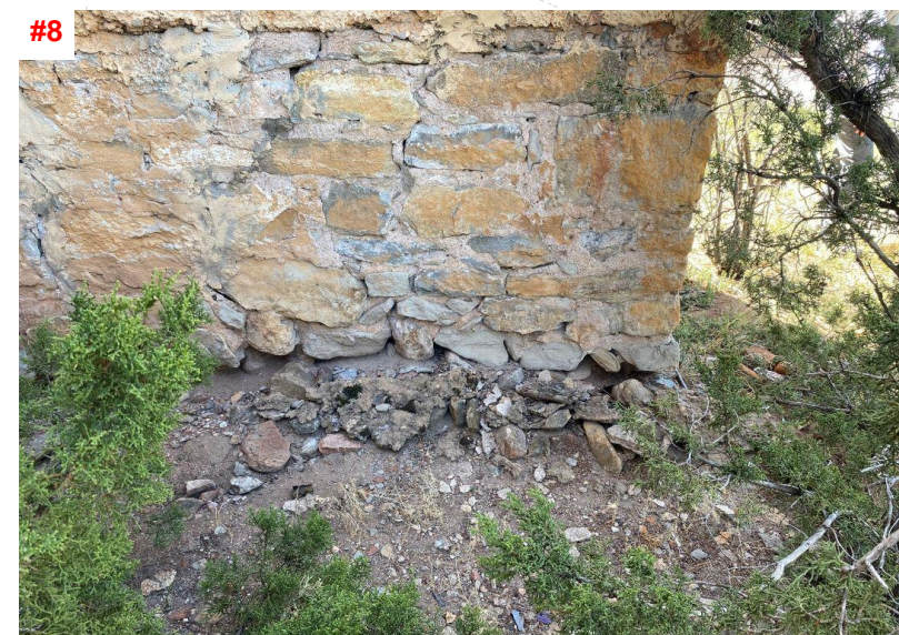
DAMAGE TO RUBBLE FOUNDATION STEM WALL
