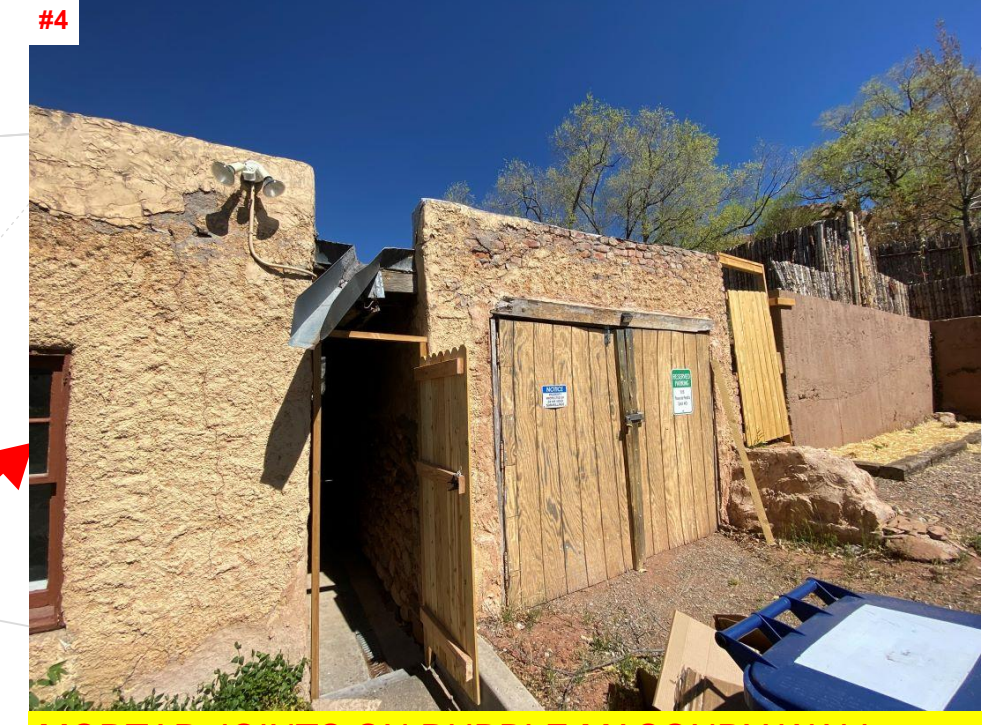
MORTAR JOINTS ON RUBBLE MASONRY WALL HAVE DE-BONDED AND HAVE COMPROMISED THE WALLS STRUCTURAL INTEGRITY.
