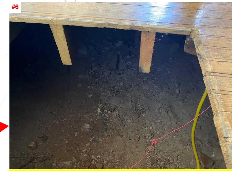
2x8 FLOOR JOISTS CUT AT OUT-OF-SERVICE GAS FLOOR HEATERS
