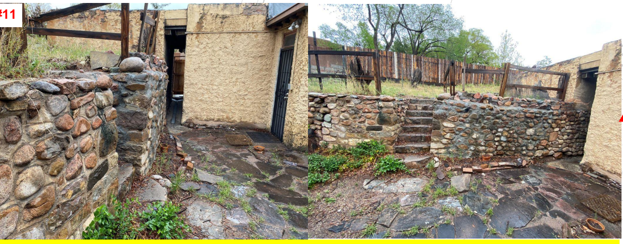
CRACK EXTENDS THROUGH ENTIRE WALL SECTION, MASONRY COURSES HAVE DE-BONDED AND THE STRUCTURAL INTEGRITY OF THE WALL HAS BEEN COMPROMISED
