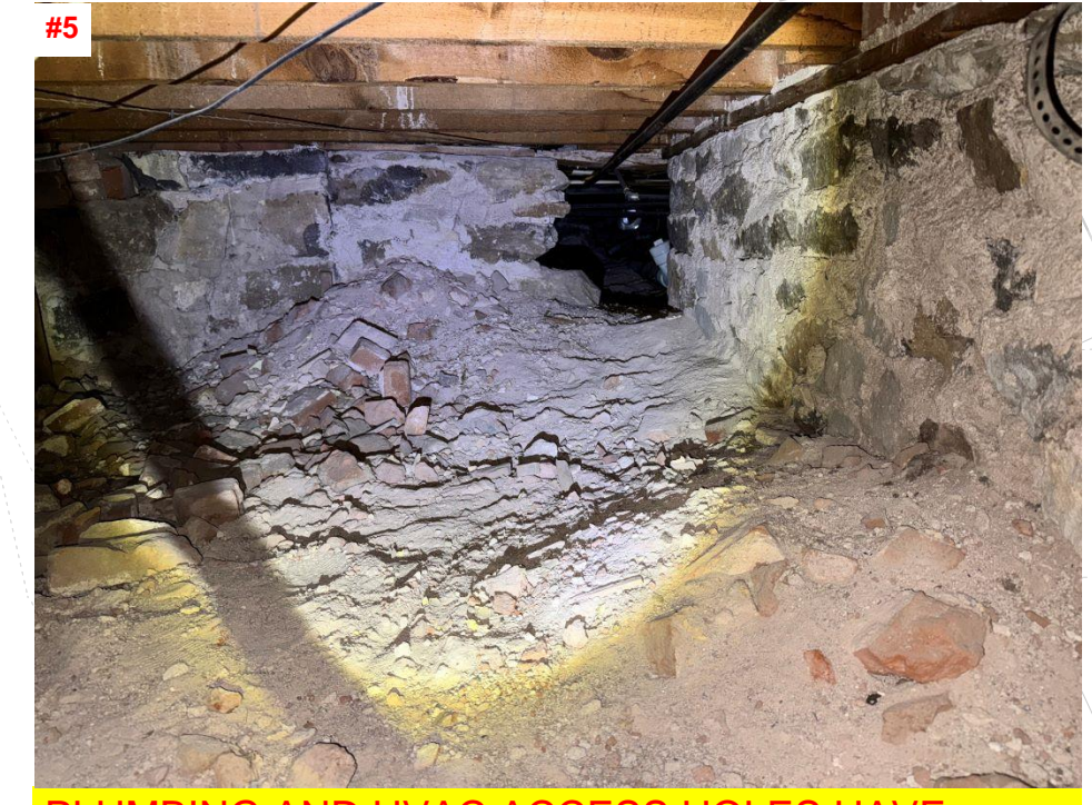
PLUMBING AND HVAC ACCESS HOLES HAVE BEEN TUNNELED THROUGH THE STONE RUBBLE STEM WALL
