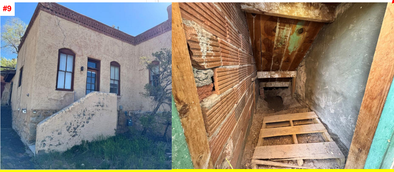
PEN-TILE STAIR WALL AND WATER DAMAGE TO WOOD STAIR FRAMING, FUNGAL DECAY OF WOOD HAS BEGUN AND HAS COMPROMISED THE STRUCTURAL SECTION
