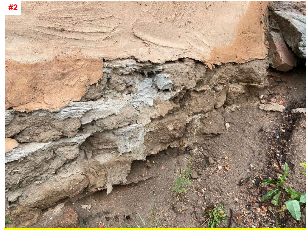
A PORTION OF THE SHED WALLS ARE CONSTRUCTED WITH ABODE. SIGNIFICANT DETERIORATION OF THE ABODE BLOCK FROM MOISTURE INTRUSION WAS OBSERVED, AND NO FOUNDATION WAS DETECTED.
