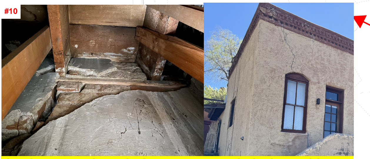
CRACK EXTENDS THROUGH ENTIRE WALL SECTION, MASONRY COURSES HAVE DE-BONDED AND THE STRUCTURAL INTEGRITY OF THE WALL HAS BEEN COMPROMISED
