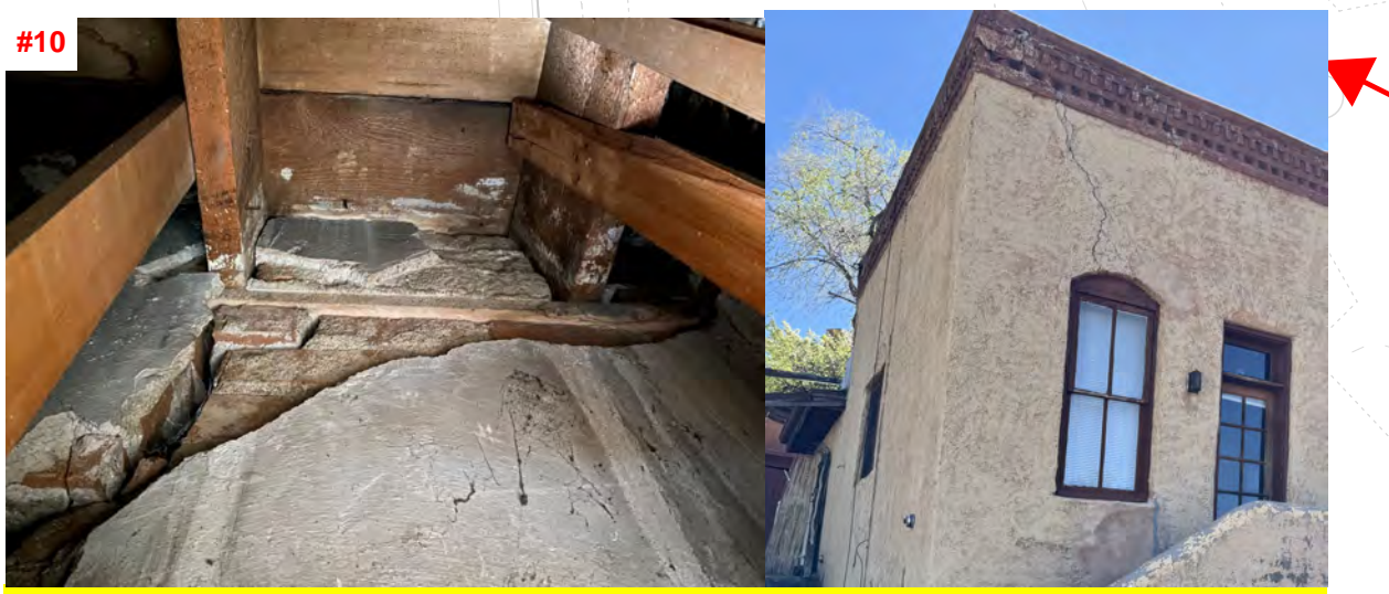
#10 CRACK EXTENDS THROUGH ENTIRE WALL SECTION, MASONRY COURSES HAVE DE-BONDED AND THE STRUCTURAL INTEGRITY OF THE WALL HAS BEEN COMPROMISED
