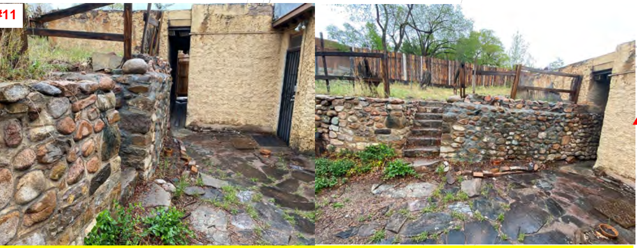
#11 CRACK EXTENDS THROUGH ENTIRE WALL SECTION, MASONRY COURSES HAVE DE-BONDED AND THE STRUCTURAL INTEGRITY OF THE WALL HAS BEEN COMPROMISED
