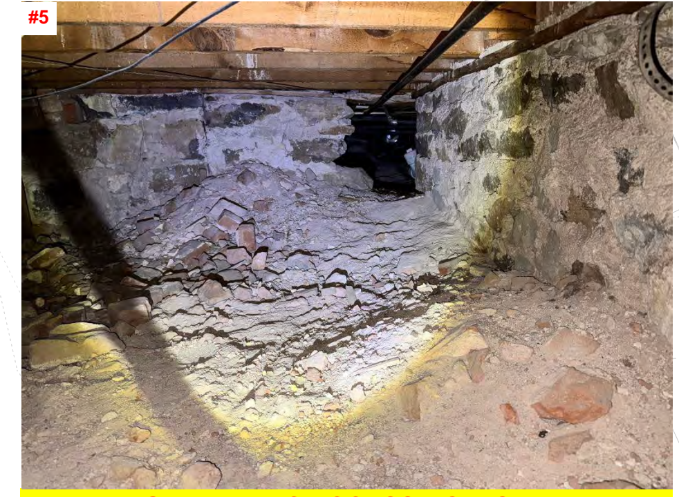
#5 PLUMBING AND HVAC ACCESS HOLES HAVE BEEN TUNNELED THROUGH THE STONE RUBBLE STEM WALL
