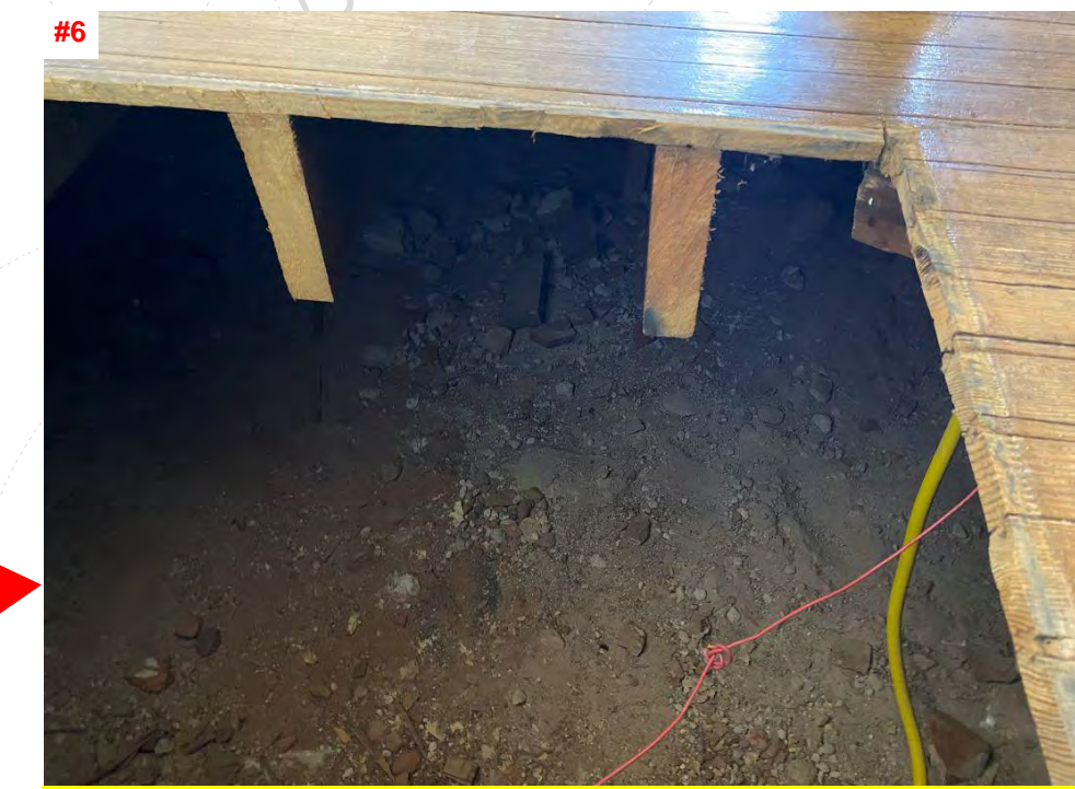
#6 2x8 FLOOR JOISTS CUT AT OUT-OF-SERVICE GAS FLOOR HEATERS
