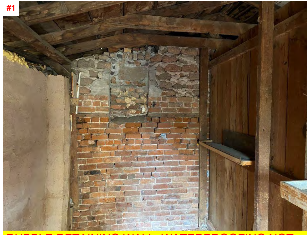
#1 RUBBLE RETAINING WALL, WATERPROOFING NOT PRESENT AND DETERIORATION PRESENTS ON EXTERIOR & INTERIOR FACES.
