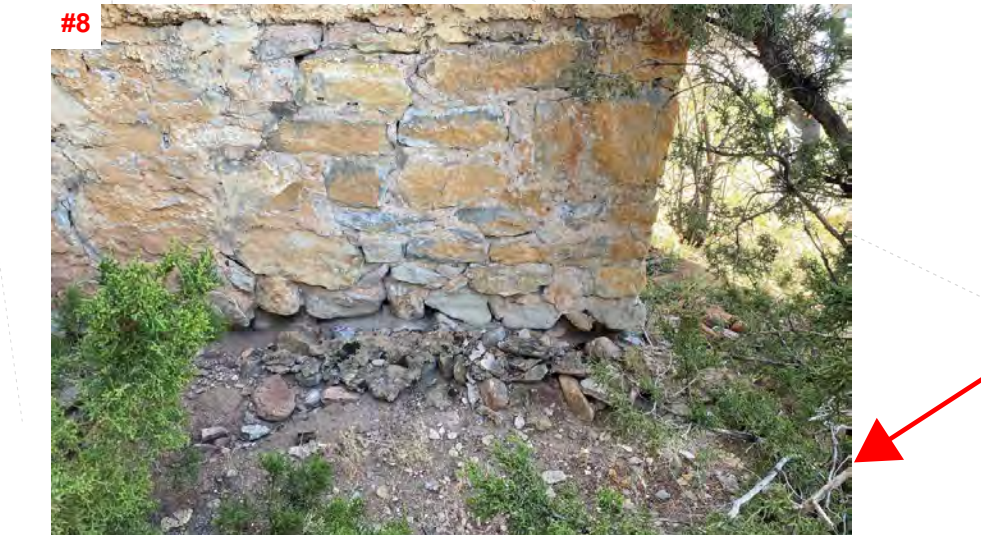
#8 DAMAGE TO RUBBLE FOUNDATION STEM WALL
