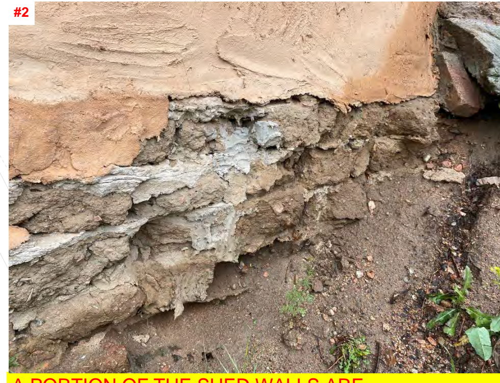
#2 A PORTION OF THE SHED WALLS ARE CONSTRUCTED WITH ABODE. SIGNIFICANT DETERIORATION OF THE ADOBE BLOCK FROM MOISTURE INTRUSION WAS OBSERVED
