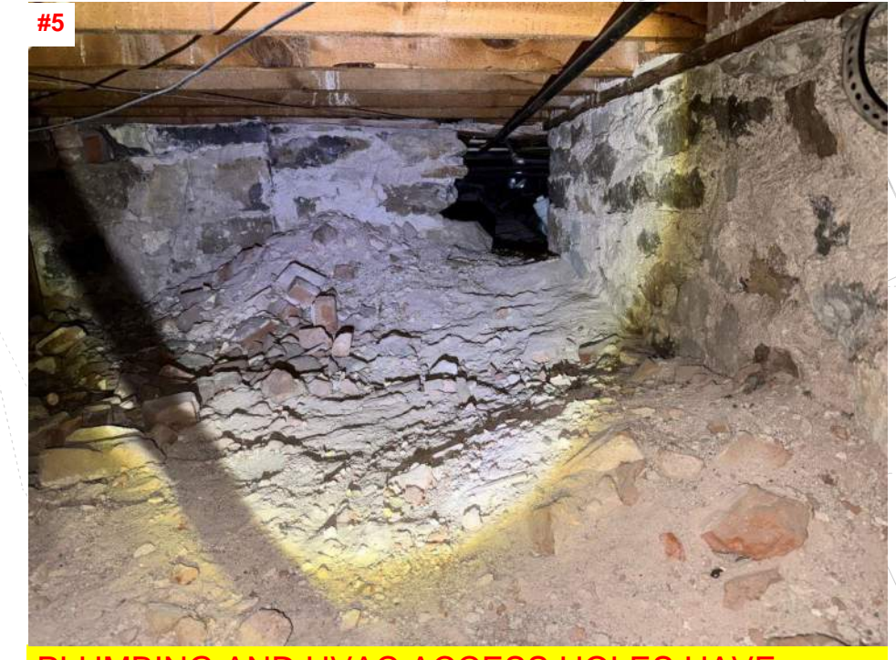
#5 PLUMBING AND HVAC ACCESS HOLES HAVE BEEN TUNNELED THROUGH THE STONE RUBBLE STEM WALL
