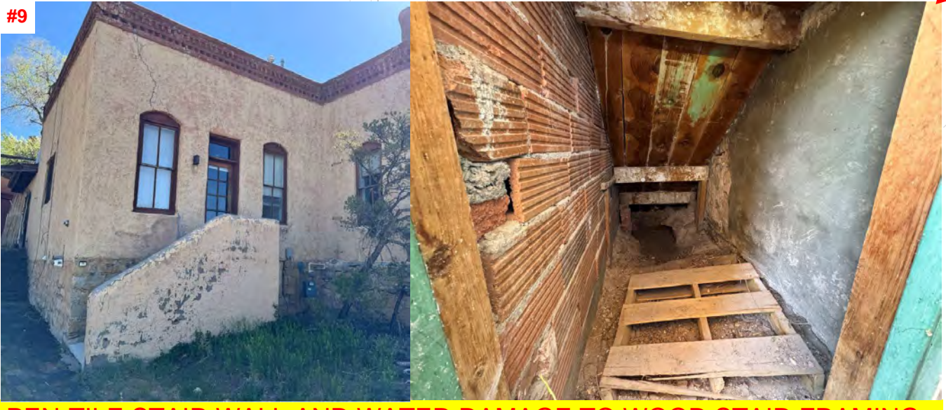
#9 PEN-TILE STAIR WALL AND WATER DAMAGE TO WOOD STAIR FRAMING, FUNGAL DECAY OF WOOD HAS BEGUN AND HAS COMPROMISED THE STRUCTURAL SECTION
