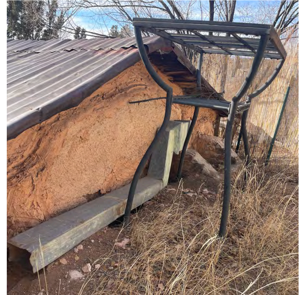
NORTH WALL IS ACTING AS A RETAINING WALL (STRUCTURAL CONCERN)
