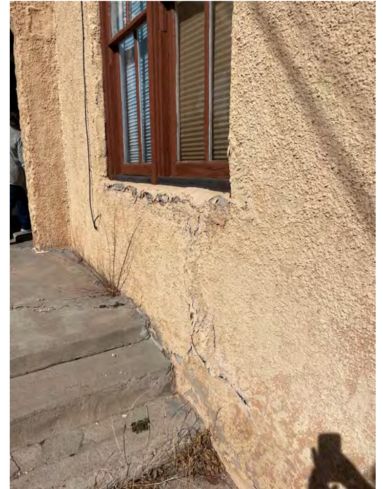
CAUSE OF CRACKS
