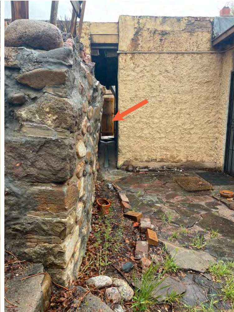
STONE RETAINING WALL (STRUCTURAL CONCERN)
