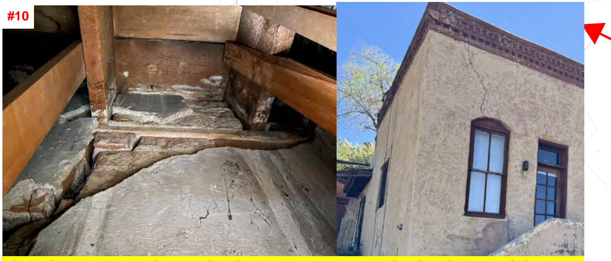
#10 CRACK EXTENDS THROUGH ENTIRE WALL SECTION, MASONRY COURSES HAVE DE-BONDED AND THE STRUCTURAL INTEGRITY OF THE WALL HAS BEEN COMPROMISED
