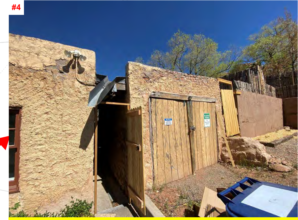
#4 MORTAR JOINTS ON RUBBLE MASONRY WALL HAVE DE-BONDED AND HAVE COMPROMISED THE WALLS STRUCTURAL INTEGRITY.
