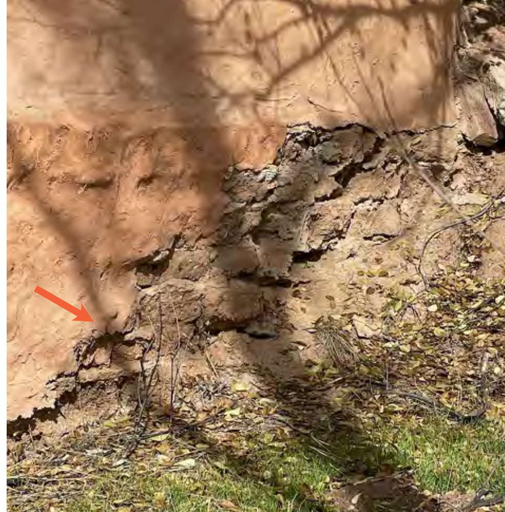
ADOBE BRICK DETERIORATING, NO FOUNDATIONS (STRUCTURAL CONCERN)
