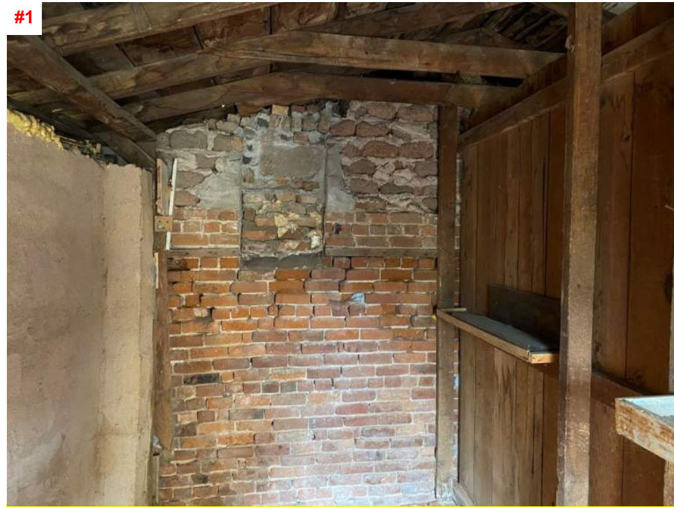
#1 RUBBLE RETAINING WALL, WATERPROOFING NOT PRESENT AND DETERIORATION PRESENTS ON EXTERIOR & INTERIOR FACES.
