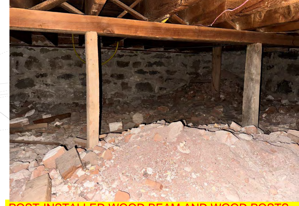
#7 POST-INSTALLED WOOD BEAM AND WOOD POSTS FOUNDED ON SOIL OR TIMBER PLANKS INSTALLED THROUGHOUT FOOTPRINT OF ORIGINAL STRUCTURE
