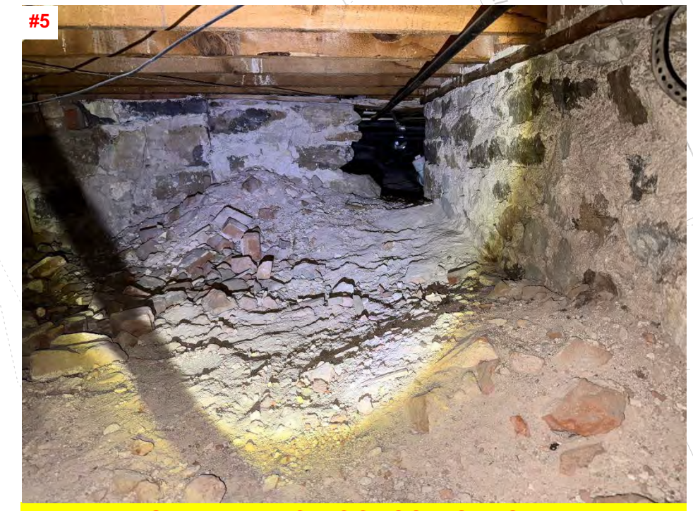
#5 PLUMBING AND HVAC ACCESS HOLES HAVE BEEN TUNNELED THROUGH THE STONE RUBBLE STEM WALL
