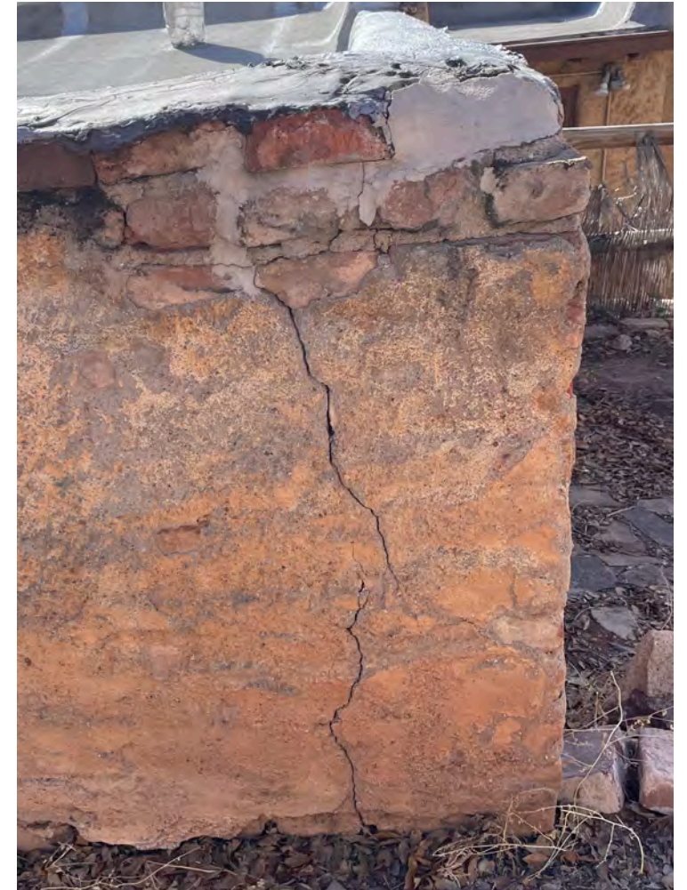
NO FOUNDATION, RETAINING AT LEAST 6' OF SOIL (STRUCTURAL CONCERN)
