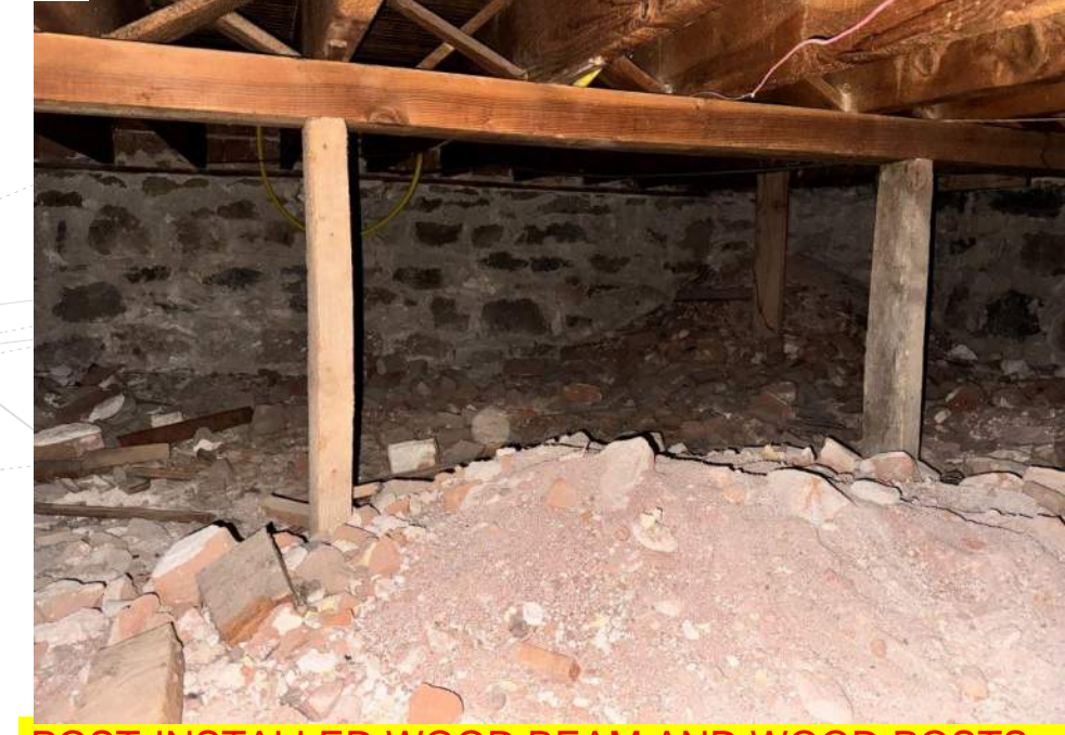
#7 POST-INSTALLED WOOD BEAM AND WOOD POSTS FOUNDED ON SOIL OR TIMBER PLANKS INSTALLED THROUGHOUT FOOTPRINT OF ORIGINAL STRUCTURE
