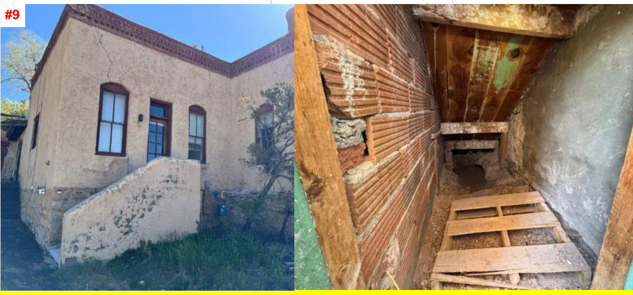
#9 PEN-TILE STAIR WALL AND WATER DAMAGE TO WOOD STAIR FRAMING, FUNGAL DECAY OF WOOD HAS BEGUN AND HAS COMPROMISED THE STRUCTURAL SECTION
