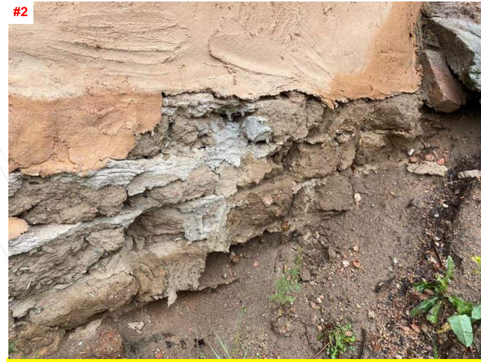
#2 A PORTION OF THE SHED WALLS ARE CONSTRUCTED WITH ADOBE. SIGNIFICANT DETERIORATION OF THE ADOBE BLOCK FROM MOISTURE INTRUSION WAS OBSERVED, AND NO FOUNDATION WAS DETECTED.
