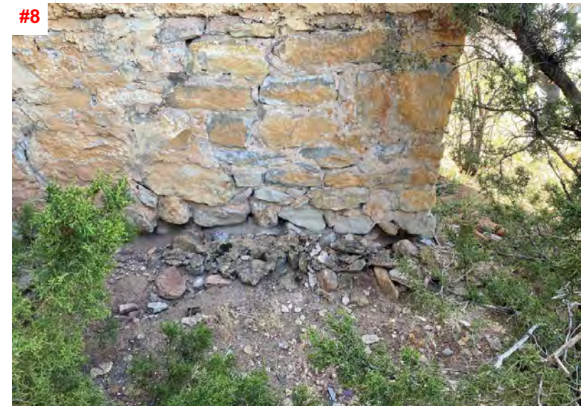
#8 DAMAGE TO RUBBLE FOUNDATION STEM WALL
