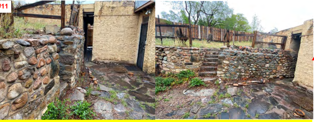
#11 CRACK EXTENDS THROUGH ENTIRE WALL SECTION, MASONRY COURSES HAVE DE-BONDED AND THE STRUCTURAL INTEGRITY OF THE WALL HAS BEEN COMPROMISED
