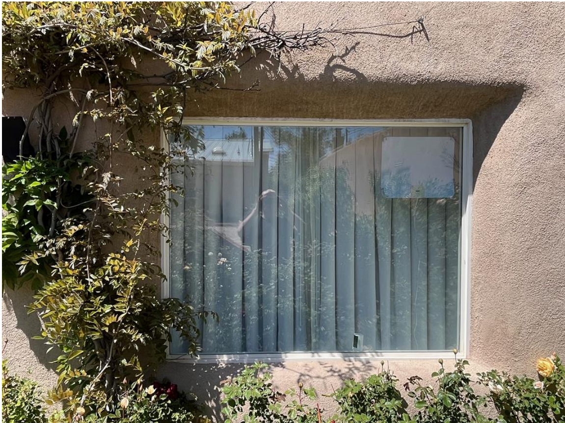
Photo 5: South elevation. Window set in original garage door opening. Camera facing north.
