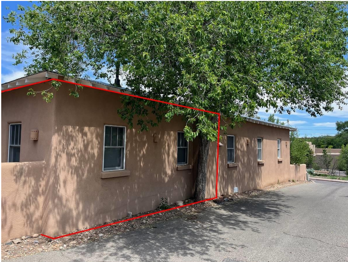
Photo 7: East elevation of 516. The red lines indicate c.1996 addition. Camera facing northwest.
