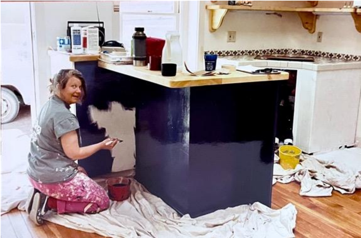
Photo 20: Room 3. Installation of kitchen at southwest corner. Camera facing southwest. Courtesy of Heidi Cost.
