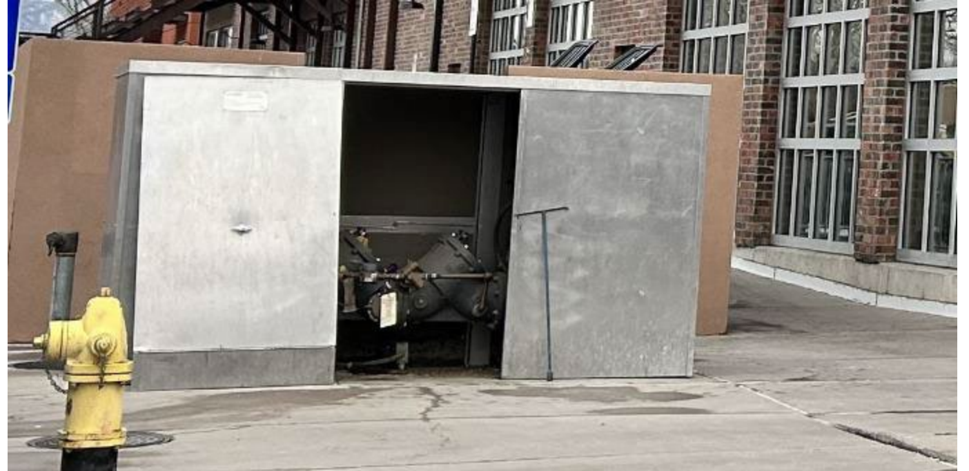
Backflow prevention assembly near Restoration Pizza in railyard
