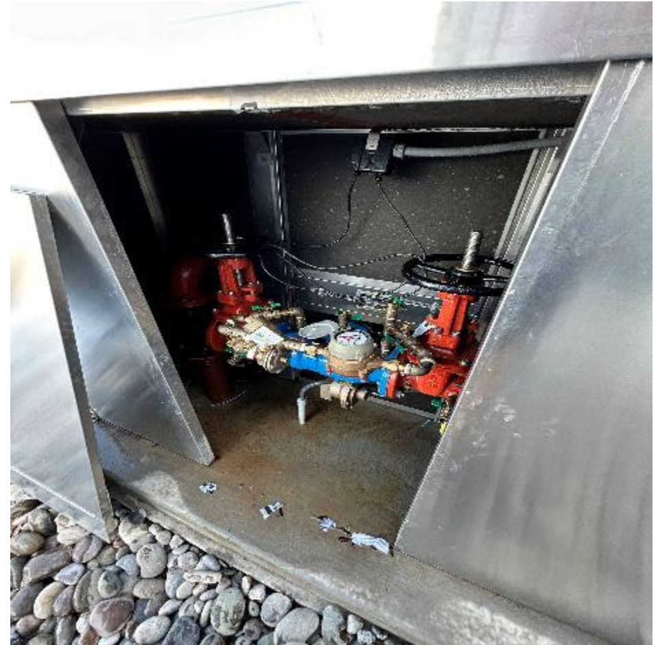
Backflow prevention assembly on fire service on Shoofly
