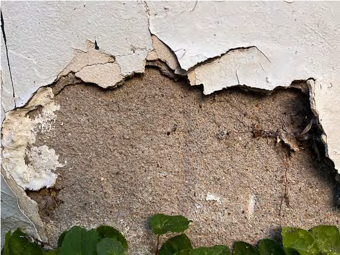
Photo 19: East elevation. Damaged stucco.
