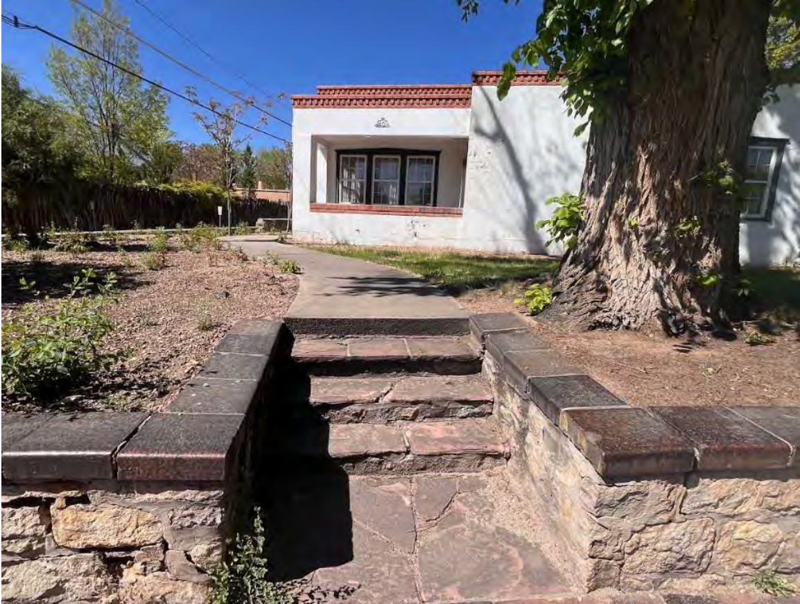
Photo 25: : South (front) retaining wall. Glazed tile coping and entry steps. Camera facing north.
