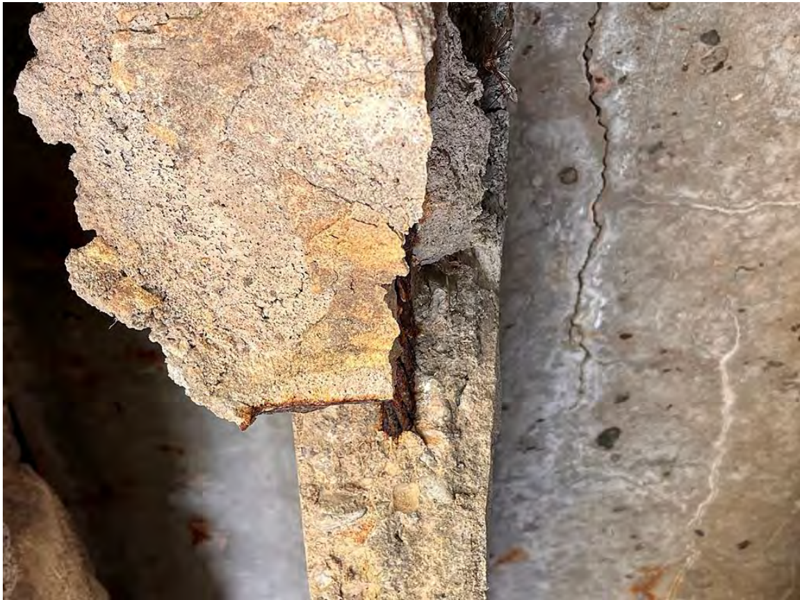
Photo 12: Deterioration to structural members, including severe delamination and exposed rebar on the beam, along with longitudinal cracking and efflorescence across the slab.
