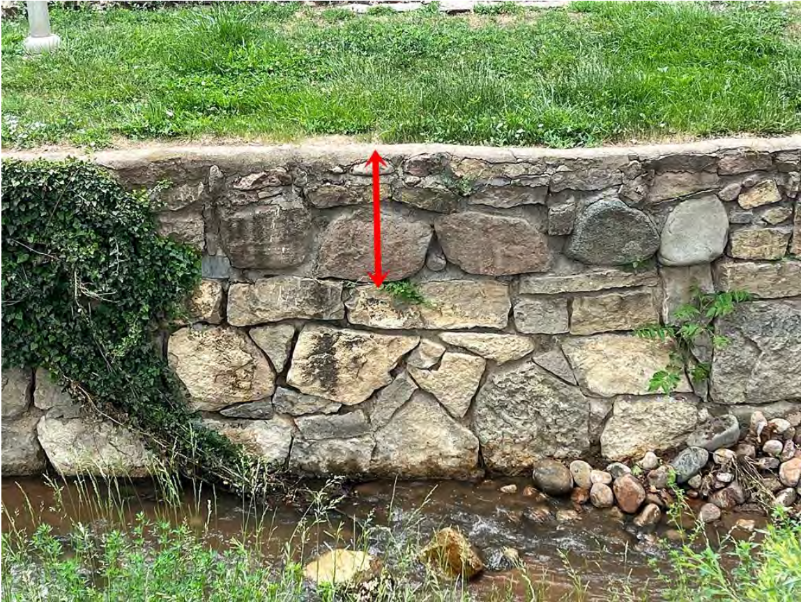
Figure 4: Contemporary photograph showing where the river retaining walls were extended in the early 1950s to create the Santa Fe River Park.
