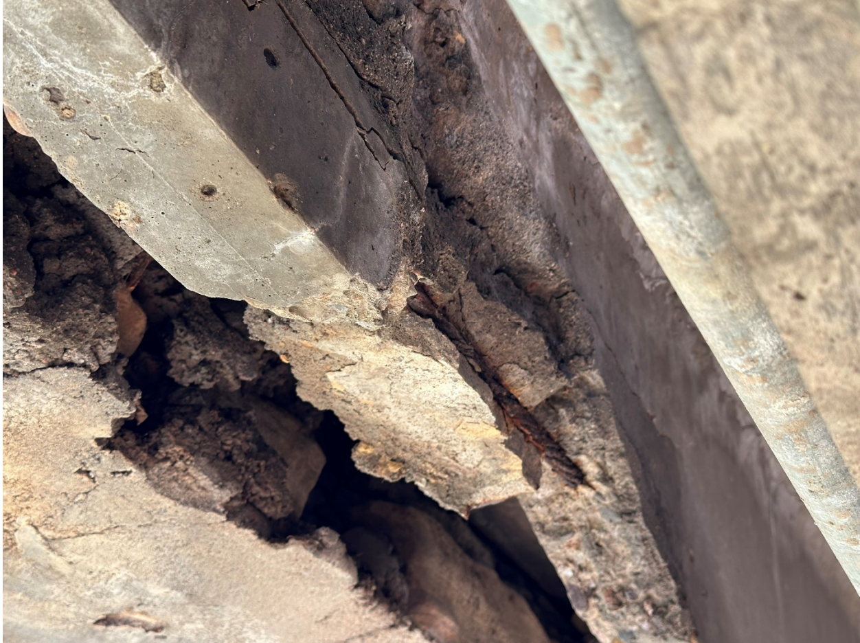
Figure 7 – Beam web spalling with exposed prestressing strand
