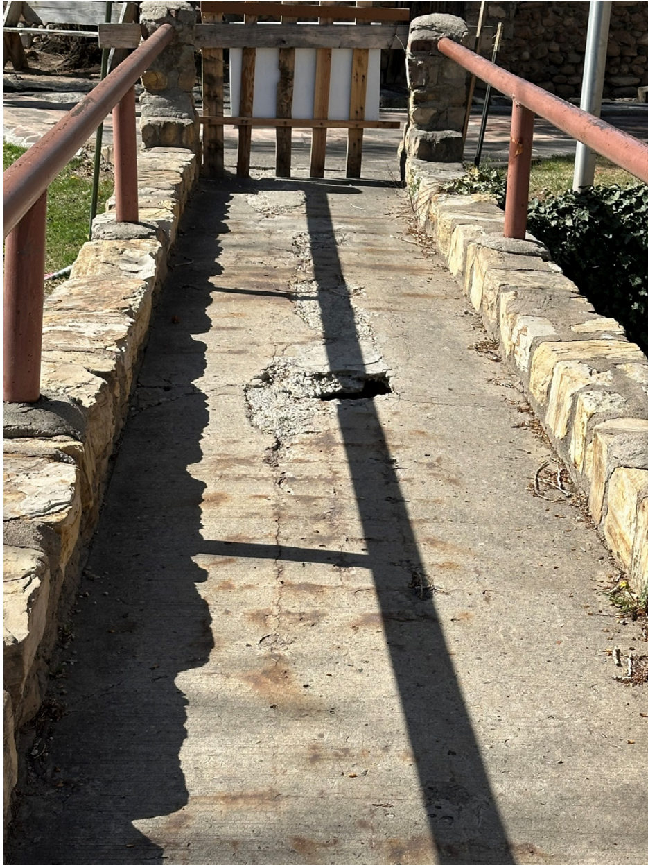
Figure 4 – Top of flange damage
