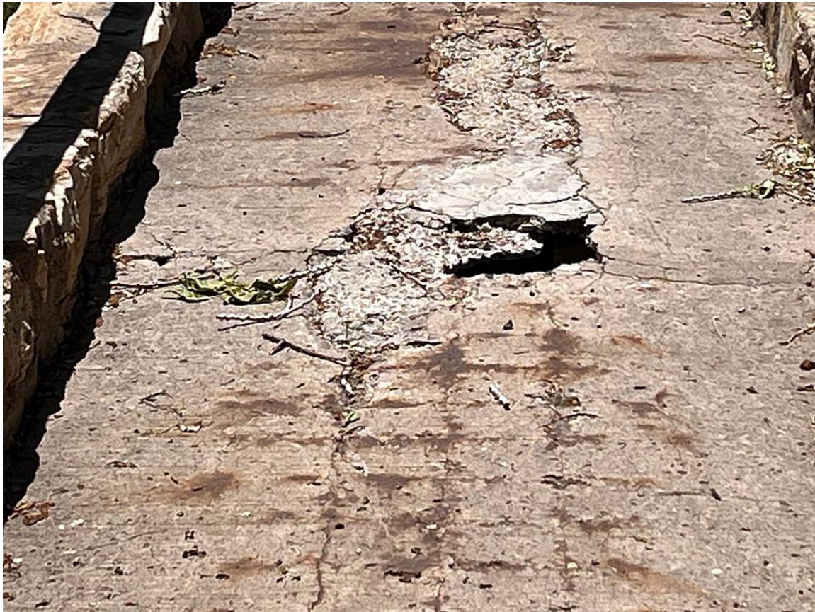
Photo 11: Deck showing punch-through, delamination, and exposed rebar mat.
