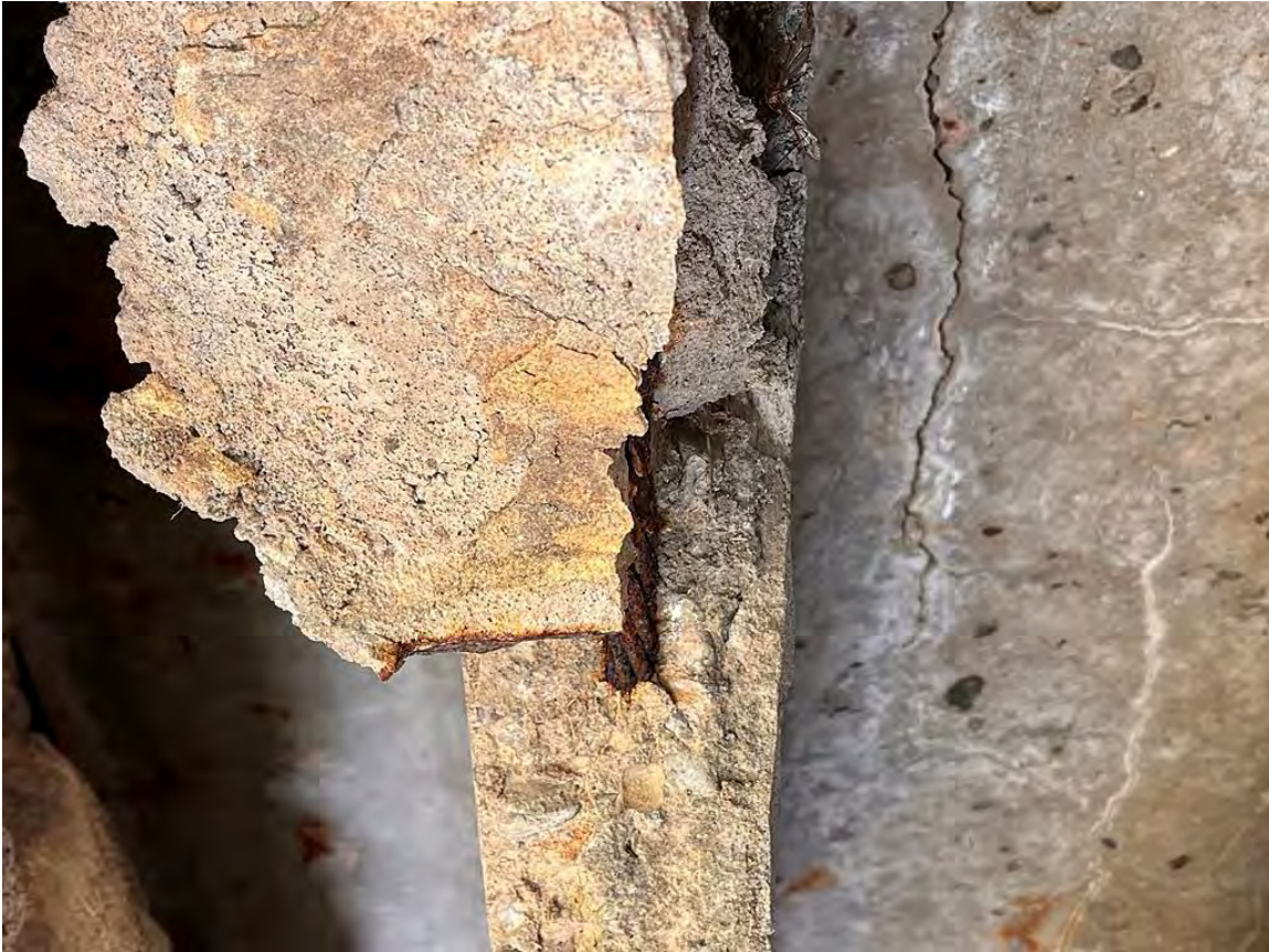
Photo 12: Deterioration to structural members, including severe delamination and exposed rebar on the beam, along with longitudinal cracking and efflorescence across the slab.
