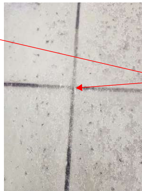
Exterior face sheet delaminating from structural grid core due to impact.
