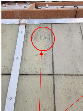
Multiple impact marks from hail stones.
