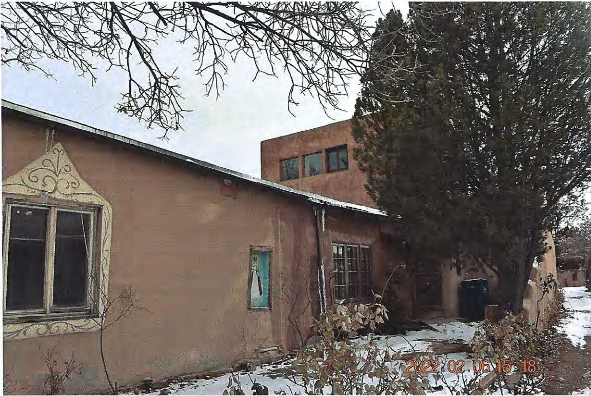
Photo 4: West elevation. Older portion, middle section; 1968 addition in background. Camera facing southeast.
