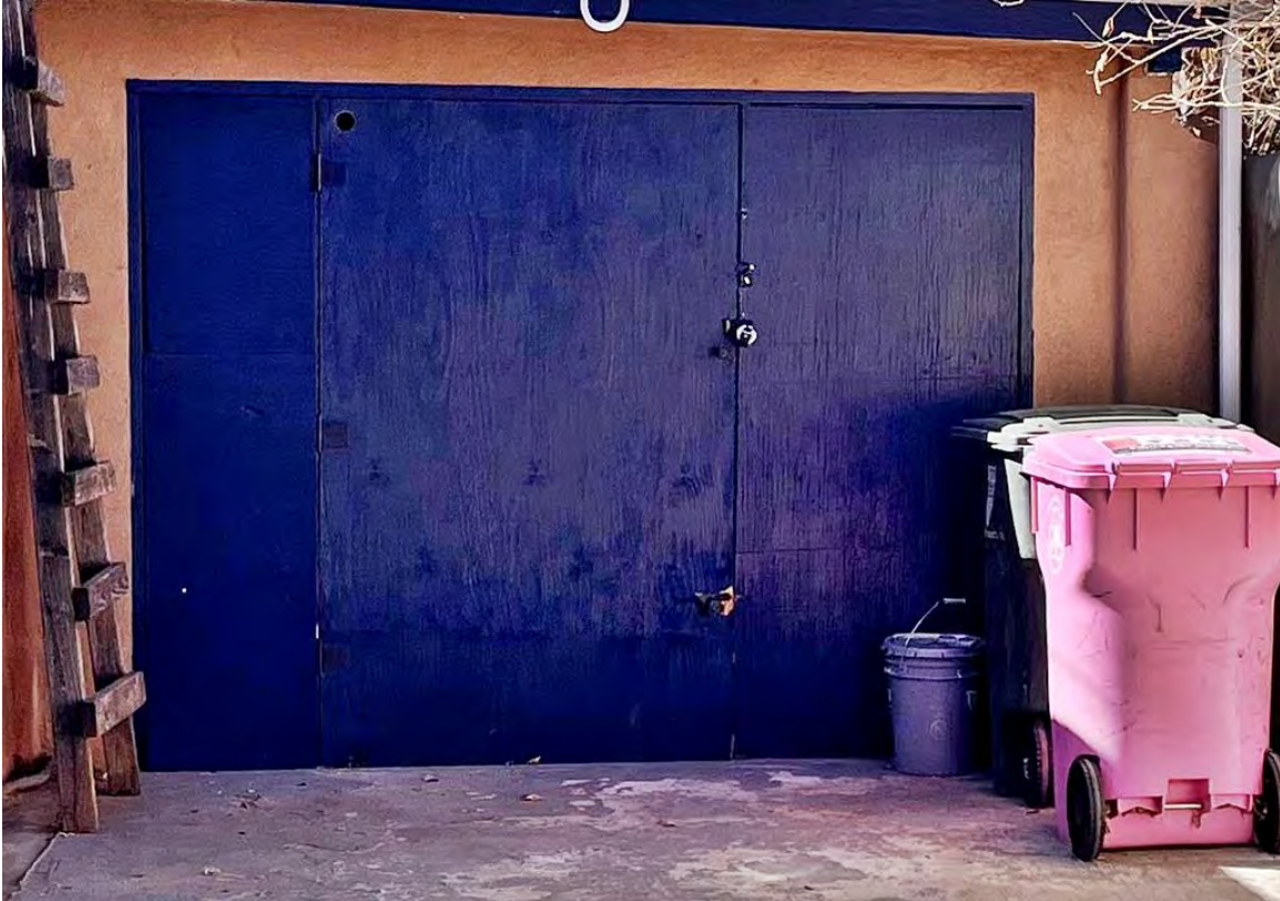
Photo 12: North elevation. Enclosed carport. Plywood doors. Camera facing west. John W. Murphey, February 27, 2025.
