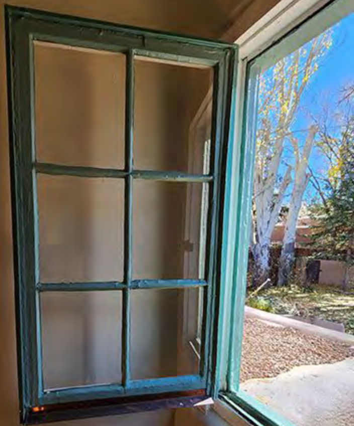
2nd Floor South Window X
