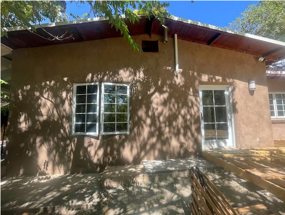
Photo 6: South elevation. Circa 1973-78 extension of west arm of historic C-shape plan. Camera facing north.
