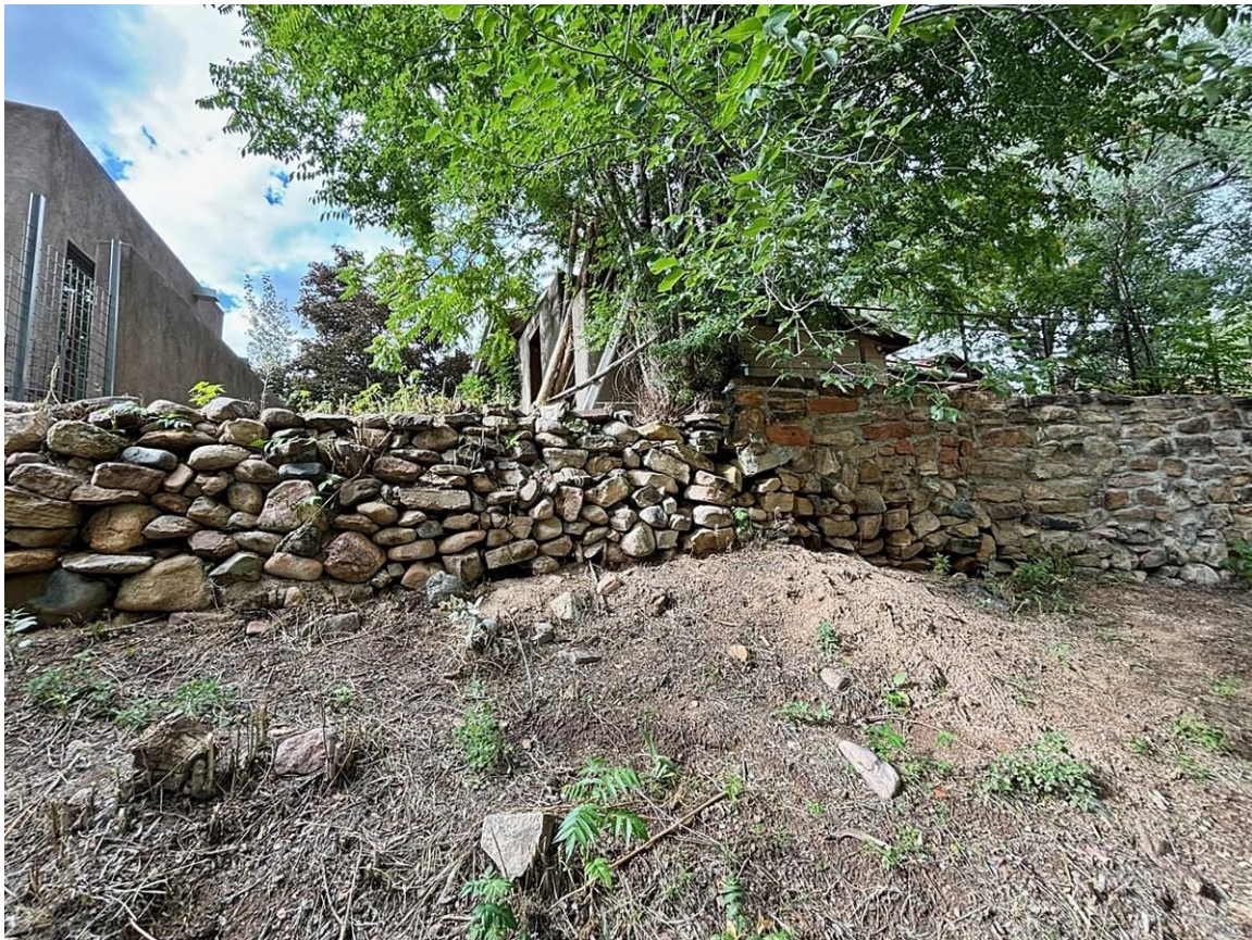
Photo 12: Upper retaining wall at west end. Camera facing north. M. Kay, August 14, 2024.
