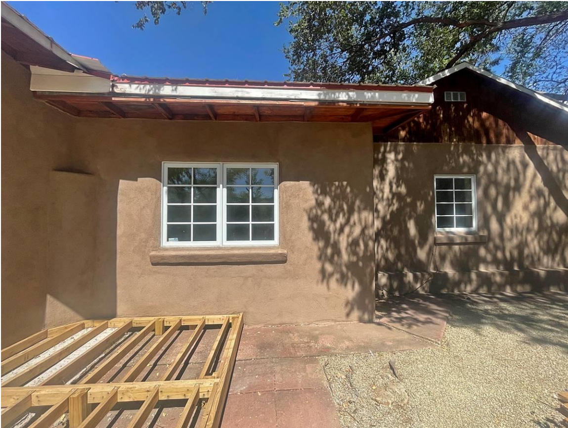
Photo 7: South elevation. Circa 1960-66 addition built across courtyard at center. Camera facing north.
