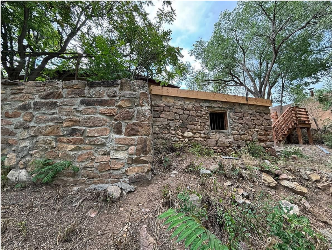
Photo 11: Upper retaining wall (left) and stone structure (right). Camera facing northeast. M. Kay, August 14, 2024.
