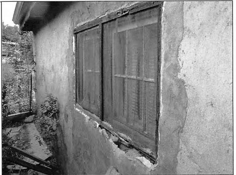
7. View south of portion of east elevation (same windows as in previous photo 6). Windows appear unaltered. Plastered adobe is in poor condition (ArcCom 07-20-06).
