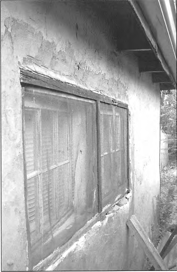
6. View north of portion of east elevation. Windows appear unaltered. Plastered adobe is in poor condition (ArcCom 07-20-06).
