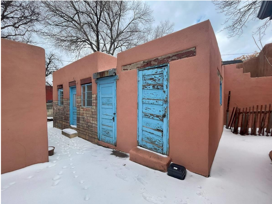
Photo 12: Storage Building. South elevation facing northwest. Right portion of building located in adjacent parcel.
