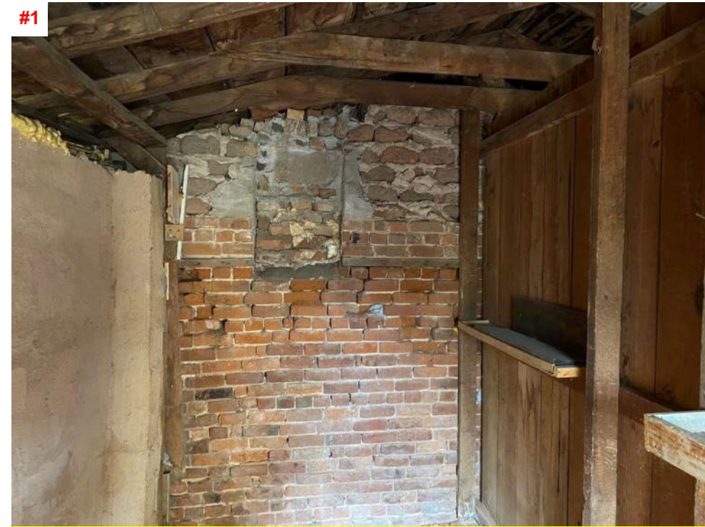
#1 RUBBLE RETAINING WALL, WATERPROOFING NOT PRESENT AND DETERIORATION PRESENTS ON EXTERIOR & INTERIOR FACES.
