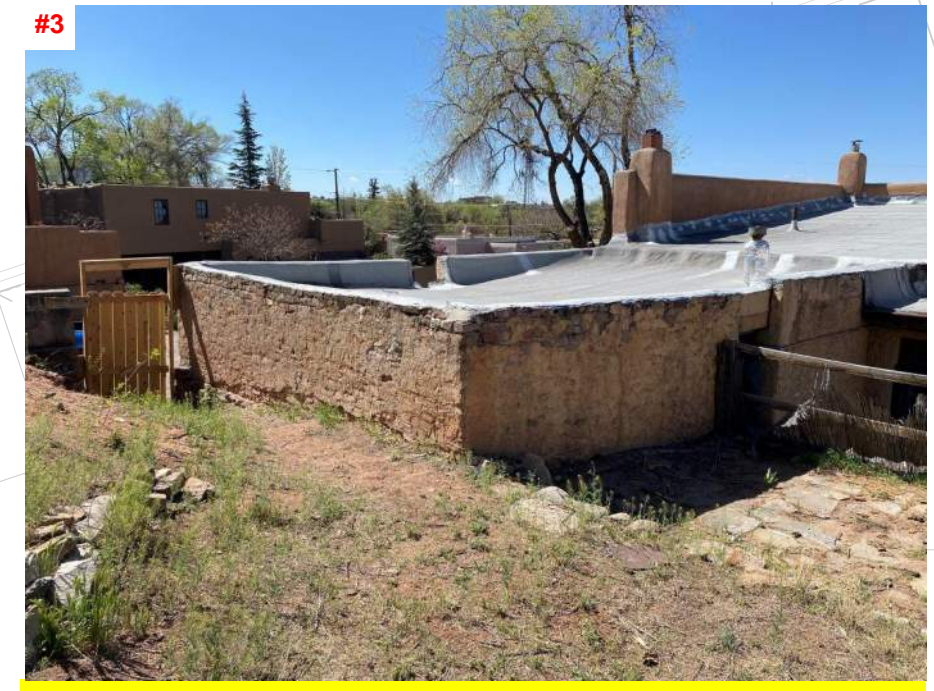
#3 RUBBLE RETAINING WALL, WATERPROOFING NOT PRESENT AND DETERIORATION PRESENTS ON EXTERIOR. THE WALL IS ALSO CONSTRUCTED WITH NON-STANDARD MASONRY MATERIAL AND PRACTICES
