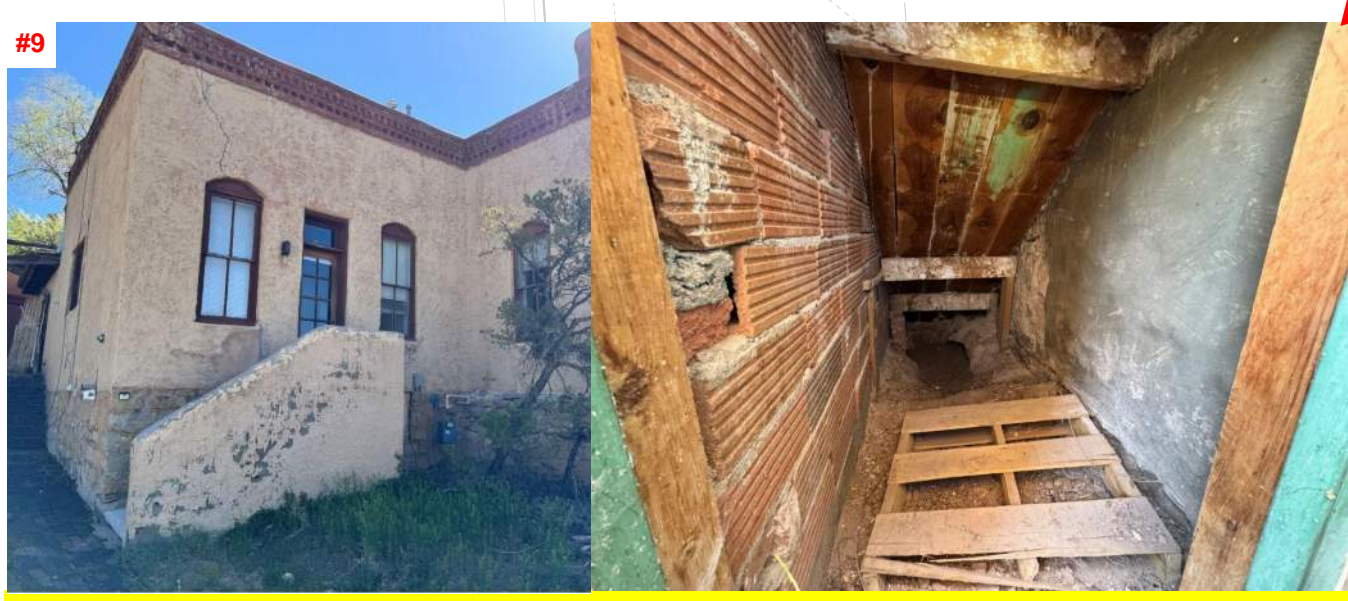
#9 PEN-TILE STAIR WALL AND WATER DAMAGE TO WOOD STAIR FRAMING, FUNGAL DECAY OF WOOD HAS BEGUN AND HAS COMPROMISED THE STRUCTURAL SECTION
