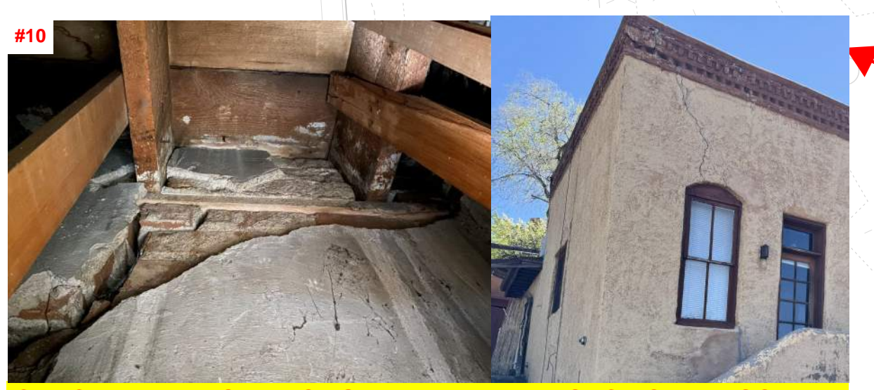
#10 CRACK EXTENDS THROUGH ENTIRE WALL SECTION, MASONRY COURSES HAVE DE-BONDED AND THE STRUCTURAL INTEGRITY OF THE WALL HAS BEEN COMPROMISED
