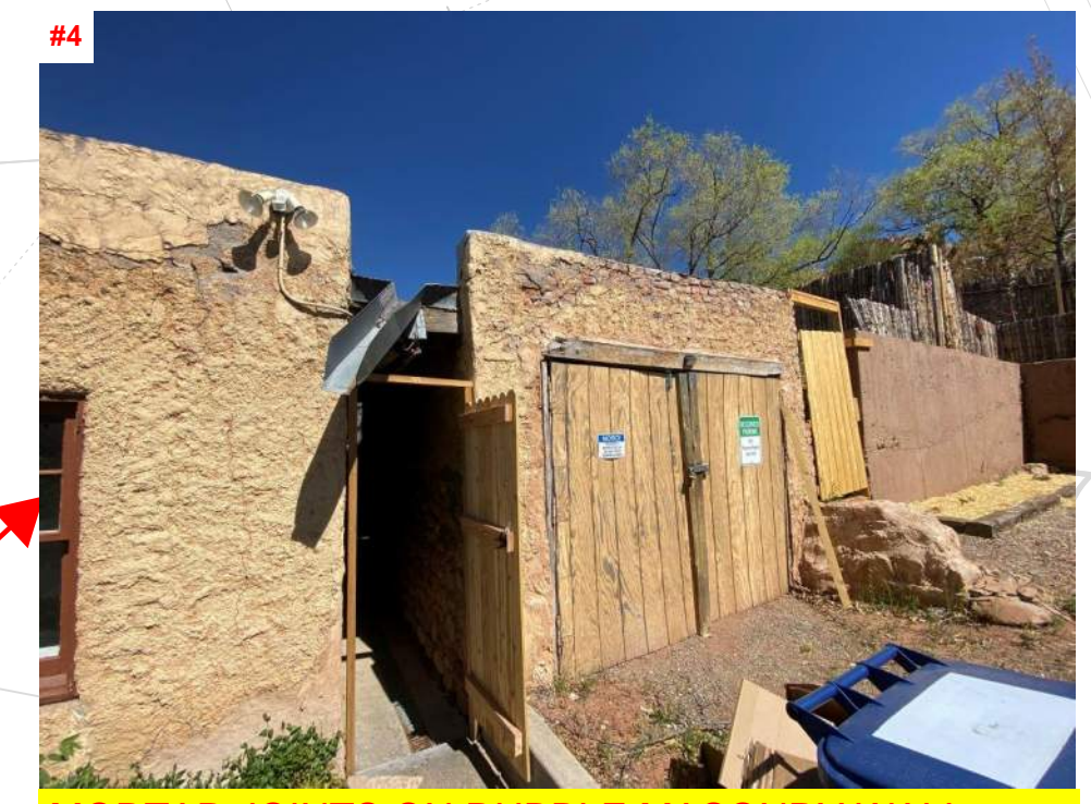
#4 MORTAR JOINTS ON RUBBLE MASONRY WALL HAVE DE-BONDED AND HAVE COMPROMISED THE WALLS STRUCTURAL INTEGRITY.
