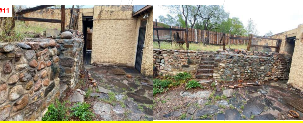
#11 CRACK EXTENDS THROUGH ENTIRE WALL SECTION, MASONRY COURSES HAVE DE-BONDED AND THE STRUCTURAL INTEGRITY OF THE WALL HAS BEEN COMPROMISED
