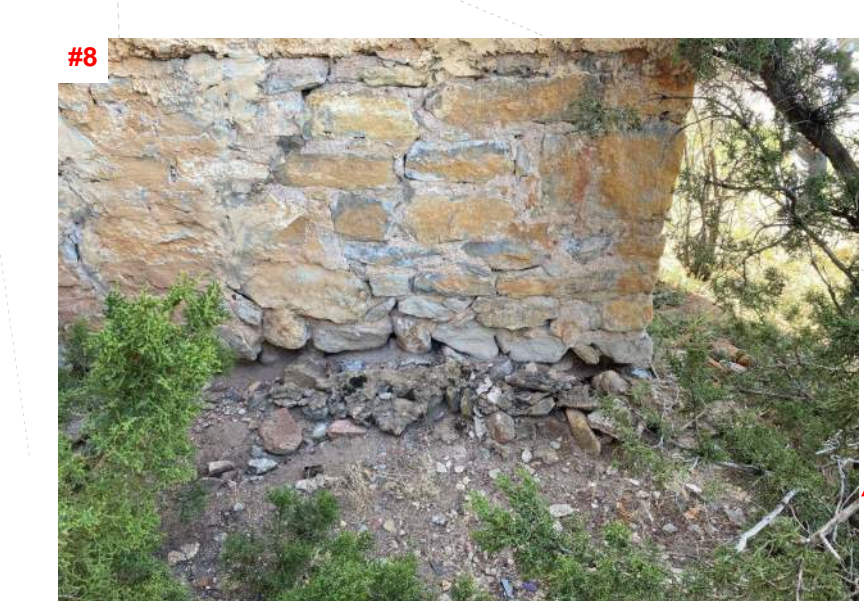
#8 DAMAGE TO RUBBLE FOUNDATION STEM WALL
