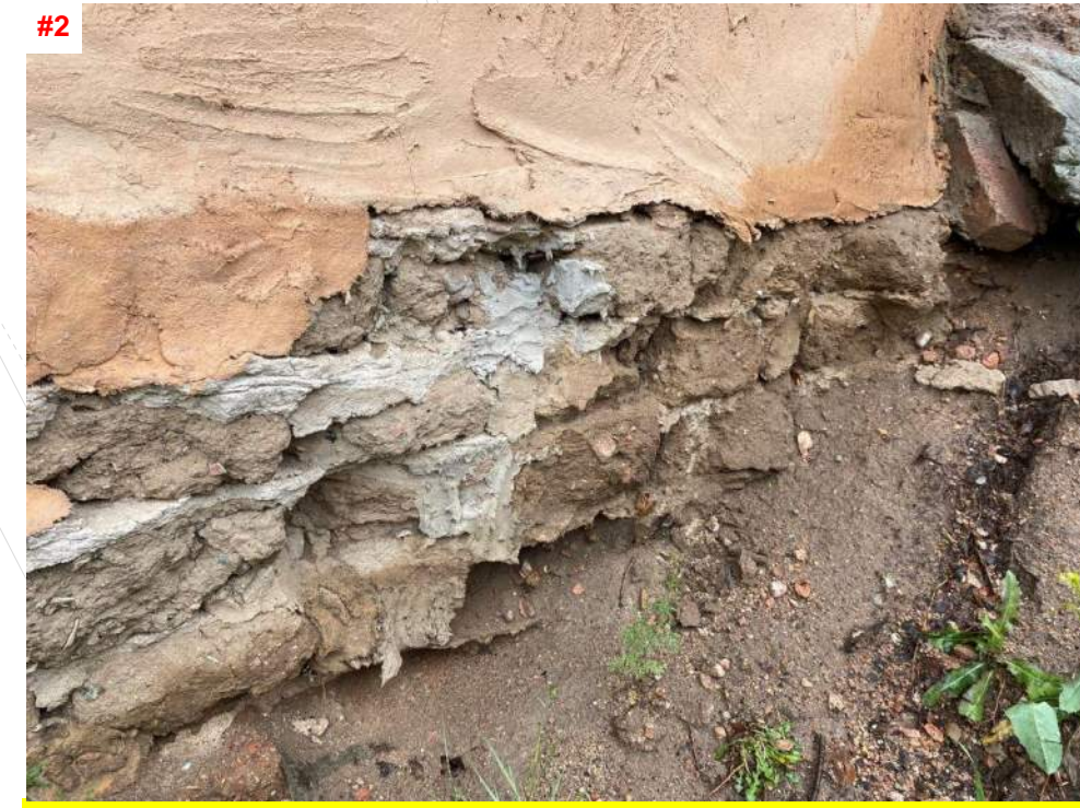
#2 A PORTION OF THE SHED WALLS ARE CONSTRUCTED WITH ADOBE. SIGNIFICANT DETERIORATION OF THE ADOBE BLOCK FROM MOISTURE INTRUSION WAS OBSERVED, AND NO FOUNDATION WAS DETECTED.
