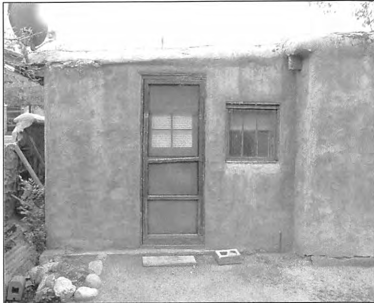
5. View south of northeast half of north elevation. Door and window appear to be unaltered (ArcCom 07-20-06).
