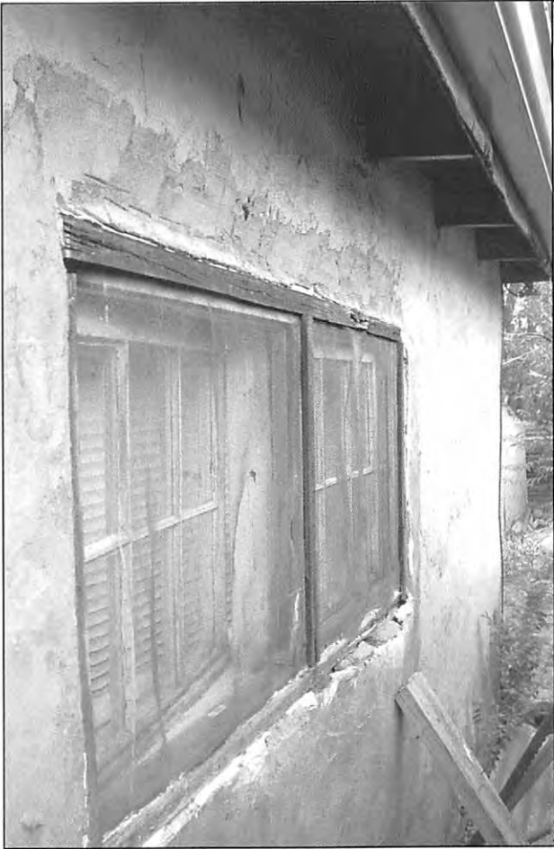
6. View north of portion of east elevation. Windows appear unaltered. Plastered adobe is in poor condition (ArcCom 07-20-06).
