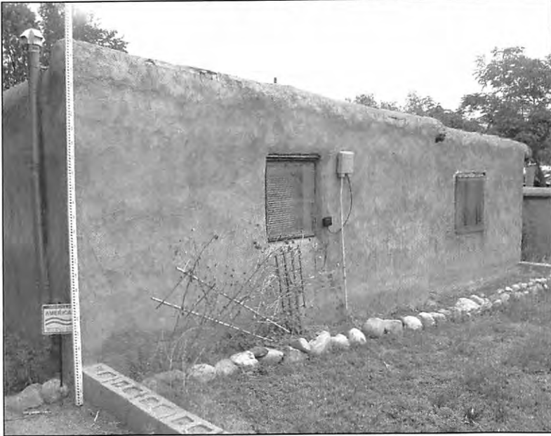
4. View northeast of south elevation. Concrete block stem wall is a structural, post-1958 alteration . Elevation at southwest corner measures 2.5 meters (8.2 feet), (ArcCom 07-20-06).
