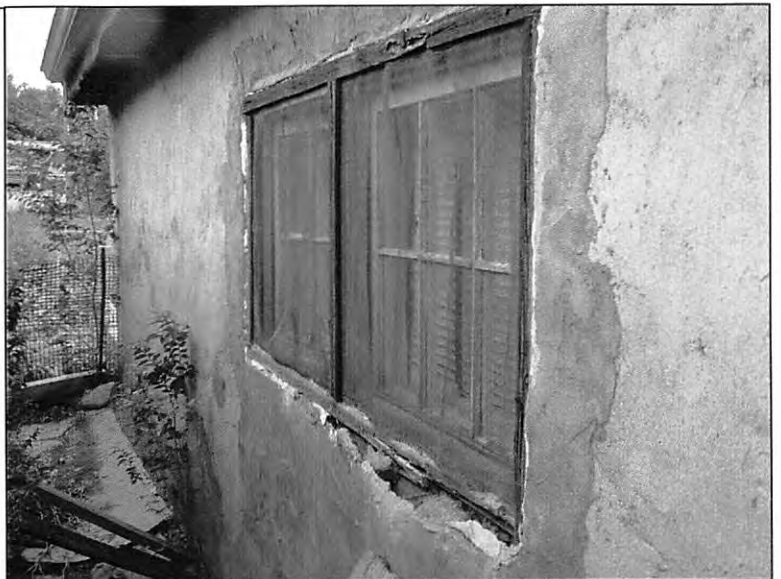
7. View south of portion of east elevation (same windows as in previous photo 6). Windows appear unaltered. Plastered adobe is in poor condition (ArcCom 07-20-06).
