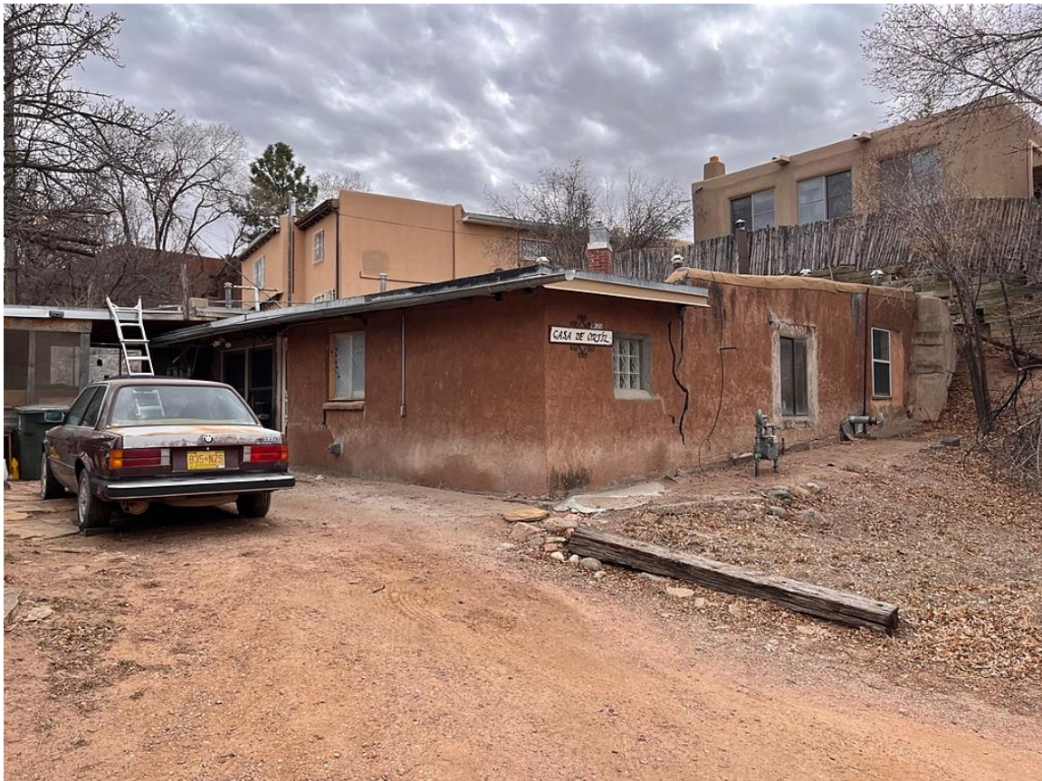
Photo 16: 537 ½ Rodriguez Street, the former José and Rosalina Ortiz House. Camera facing southeast.
