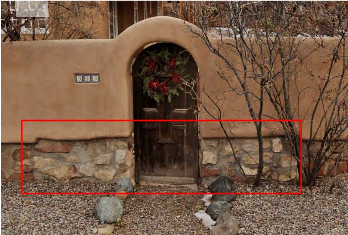
Photo 17: Altered portion of base of wall. Google Street View, December 2023.
