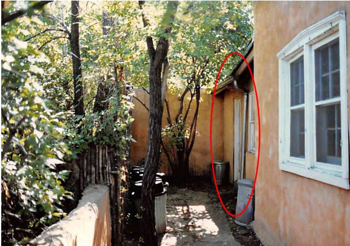
Figure 12: 1987 photograph east end of north elevation. Circle indicates change of wall position and fenestration. Compare with Photo 12. Courtesy of City of Santa Fe Historic Preservation Division.
