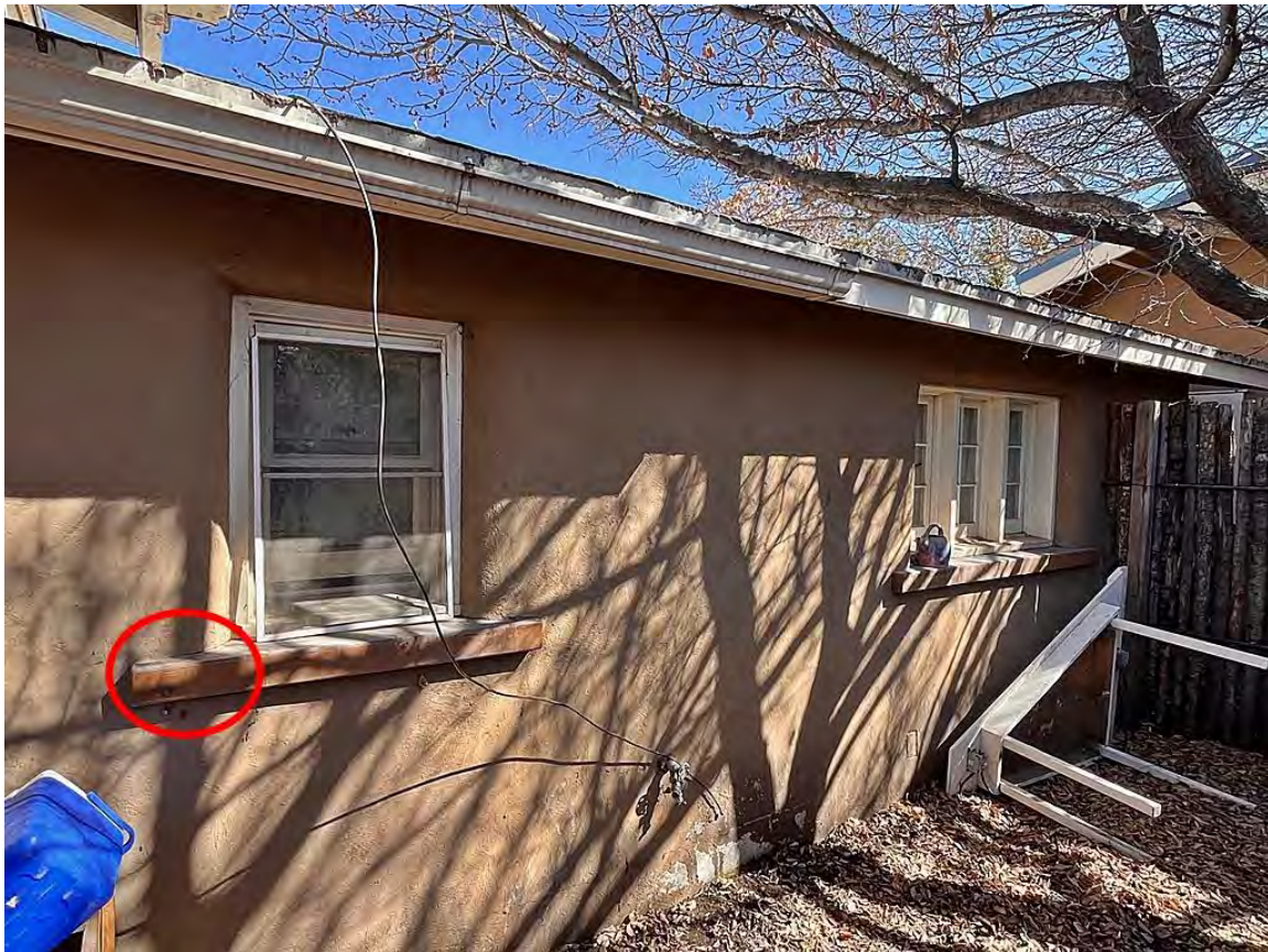
Photo 18: West elevation. South windows of post-1978 porch extension. Camera facing east. Note exaggerated wood sill.
