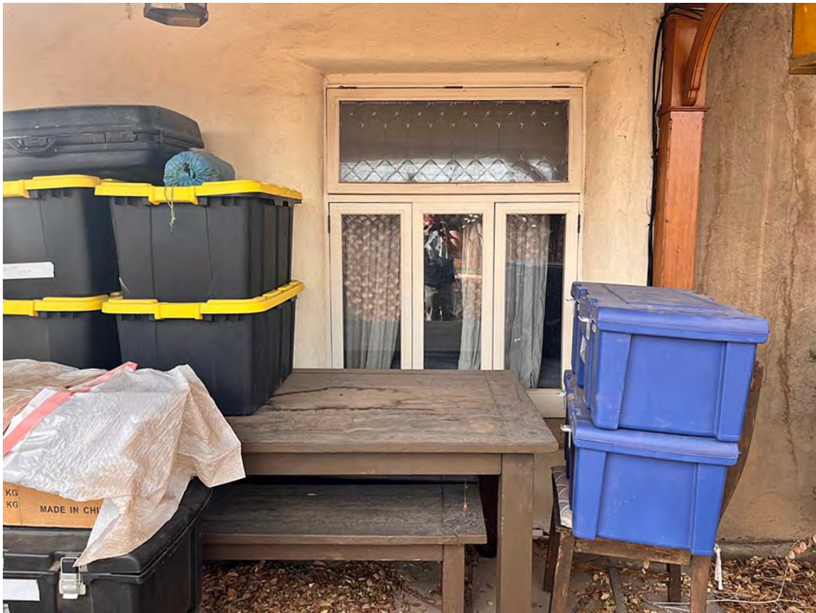
Photo 6: East elevation. North window. Camera facing west. Note inserted casement lights in lower sash.
