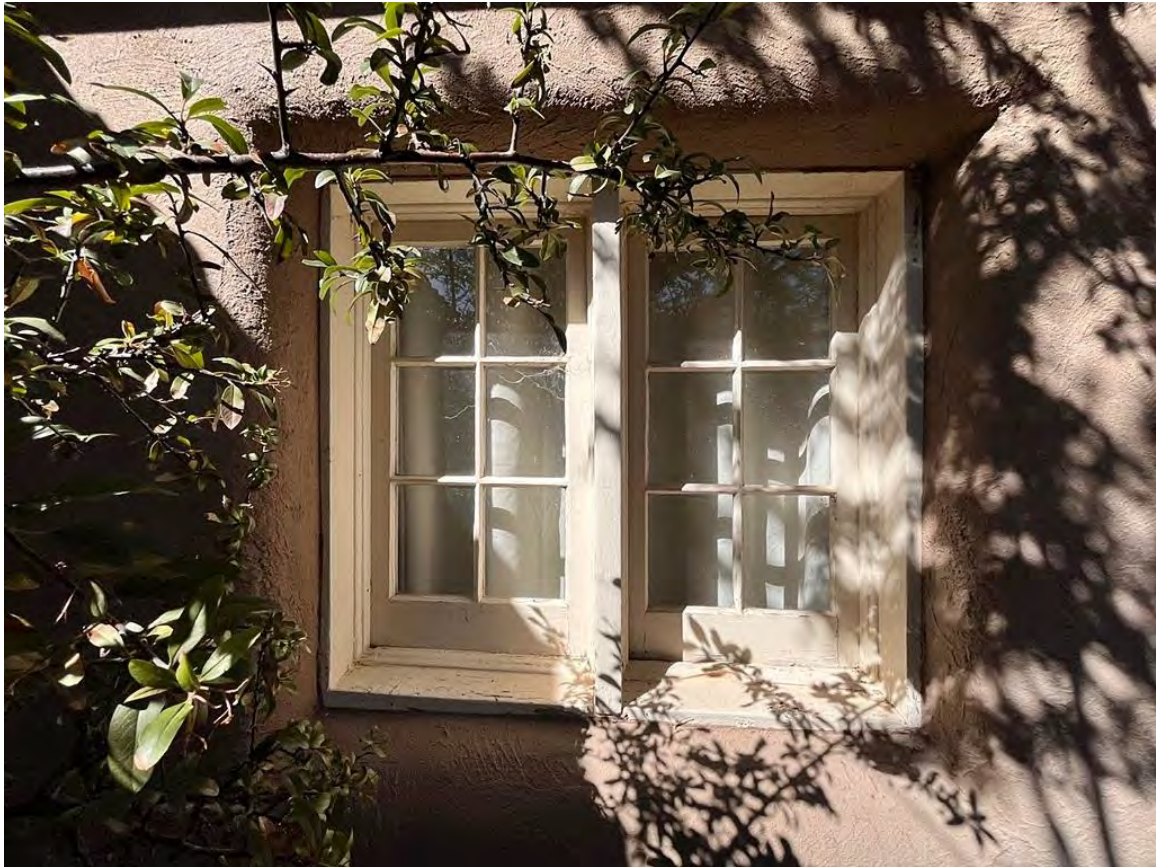
Photo 22: South elevation. Bump-out at the west end. Window detail. Camera facing northwest.
