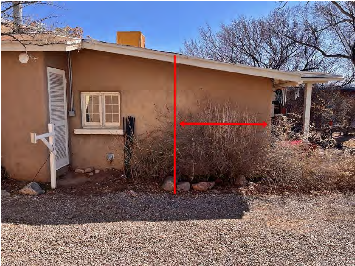
Photo 13: North elevation of enclosed and extended porch. Camera facing south. Note the porch was extended after 1978.
