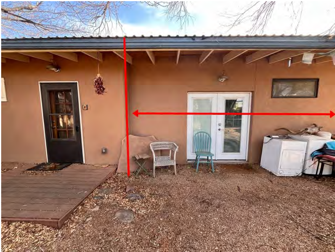
Photo 31: North elevation. The area to the right represents enclosed and extended carport. Camera facing south.
