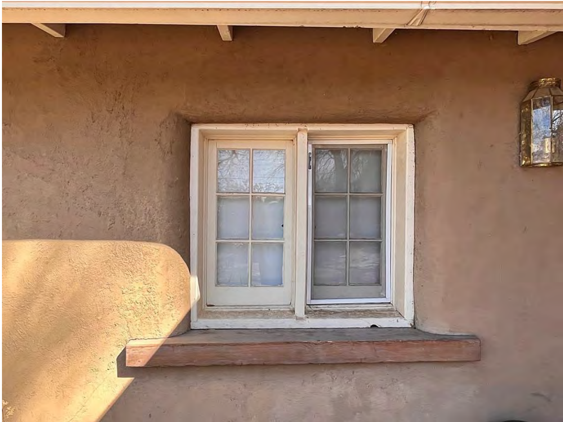
Photo 15: West elevation. North window of post-1978 porch extension. Camera facing east. Note exaggerated wood sill.
