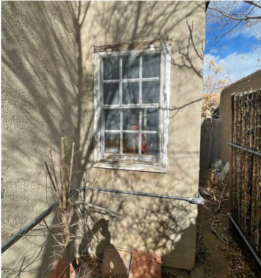
Photo 14: East elevation. Window at south side of mudroom addition. Camera facing northwest. Michael Zimber, January 29, 2025.
