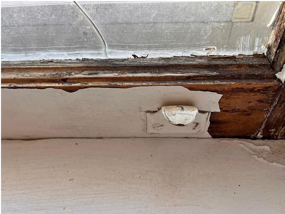
Photo 10: Deterioration of east dormer window.
