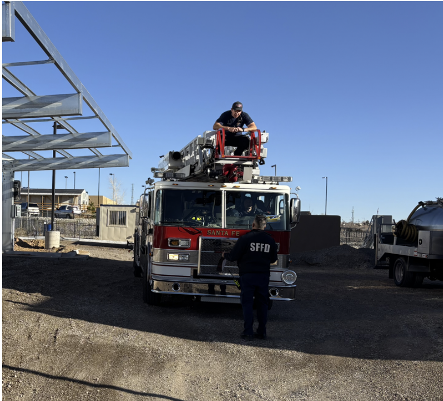
Figure 14 Fire Apparatus / Carport Structure, once panels are added fire truck circulation will be obstructed
