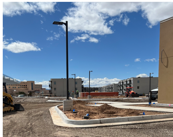
Figure 8 Installed Light Fixture
