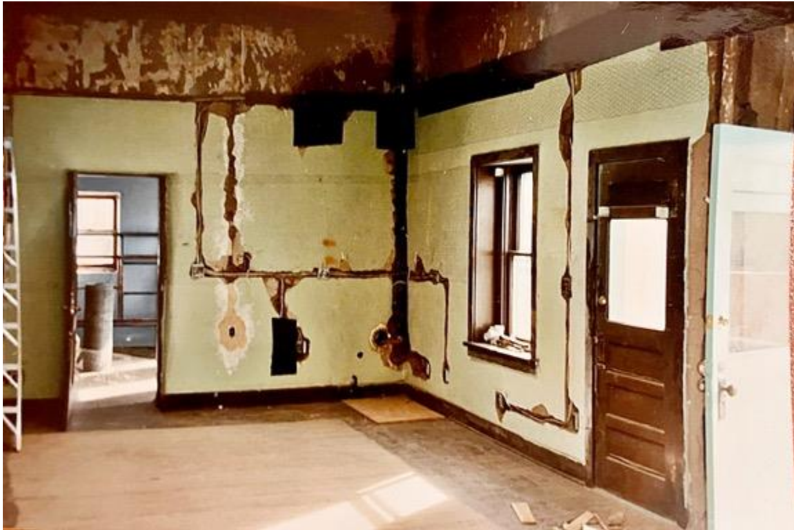
Photo 21: Room 3. 1990s renovation photograph. Camera facing southeast. Note conduit cuts in the adobe walls, removal of ceiling, and older window and door. Courtesy of Heidi Cost.
