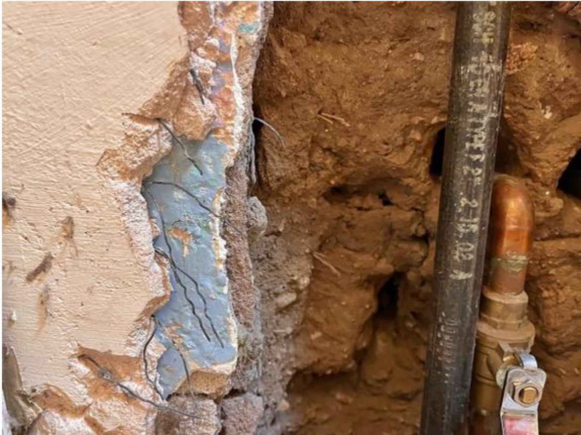
Photo 16: Exterior exposure of Room 3 at east wall, showing multiple layers of stucco and plaster.
