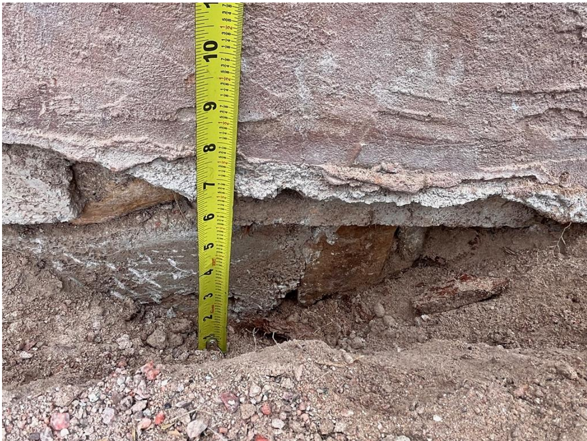
Photo 7: Exposure of foundation, consisting of poured concrete and rubble.
