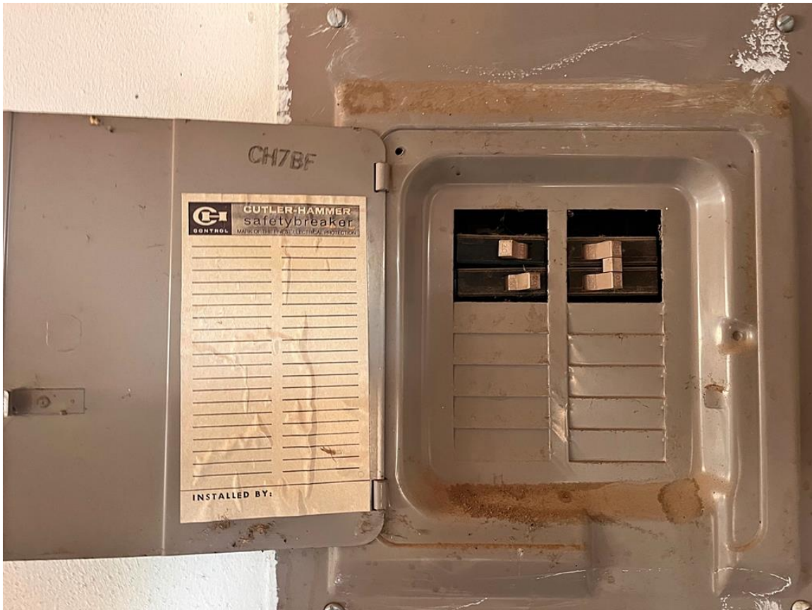
Photo 13: Breaker box on east wall.
