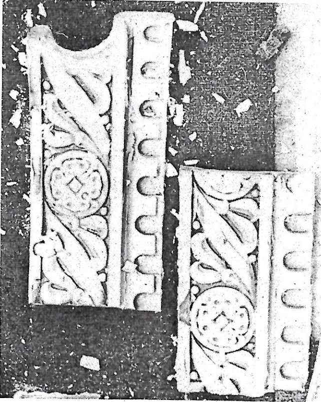
Terra Cotta Molding Lies in Pieces on Chapel Floor
