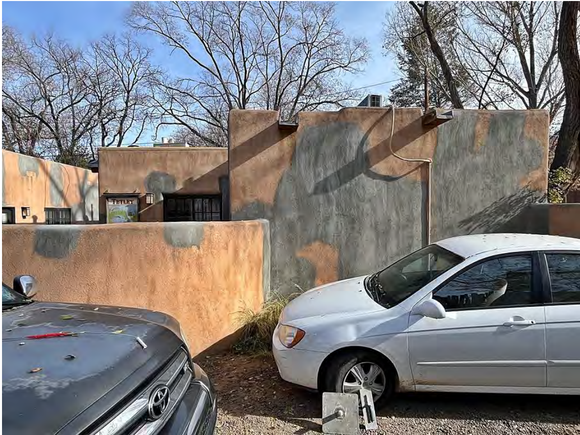
Photo 12: West elevation. Camera facing east. Note curved wall was constructed in c.2002.
